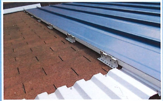
Corrugated sheeting installed at the ridge allows for continuous air flow between the existing and new roof while providing support for the panel and closure.
