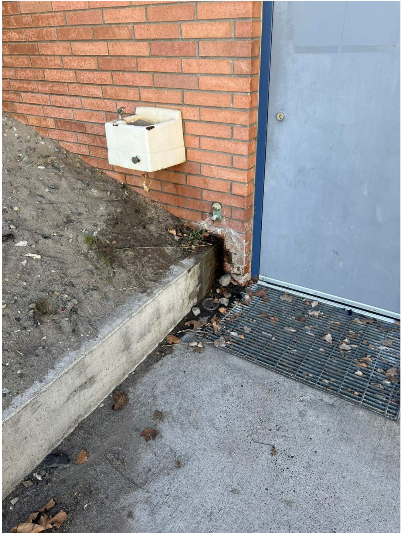
(Above: Water dripping from spicket outside North side of gymnasium door)
