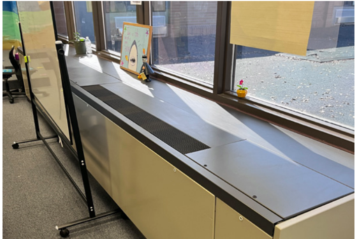
Unit ventilator and windows
