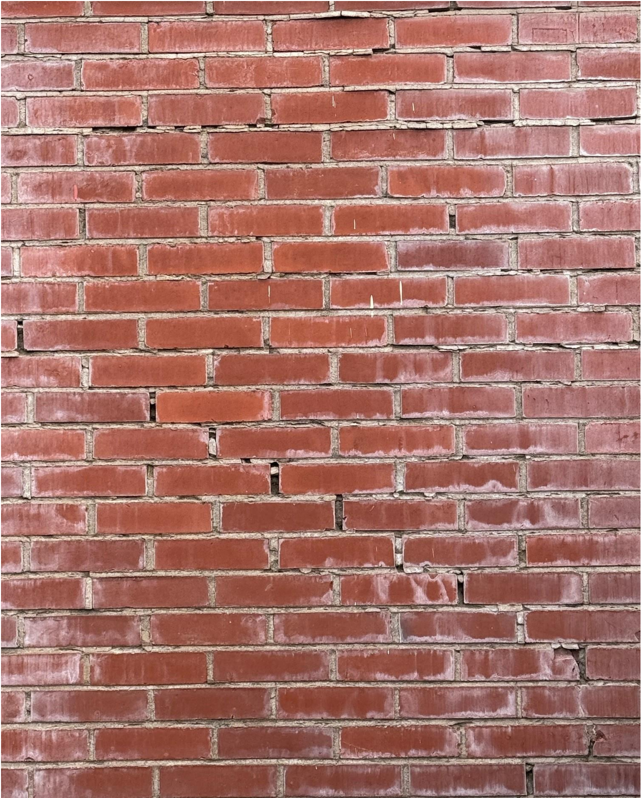
(Above: mortar damage at existing brick wall on West side)
