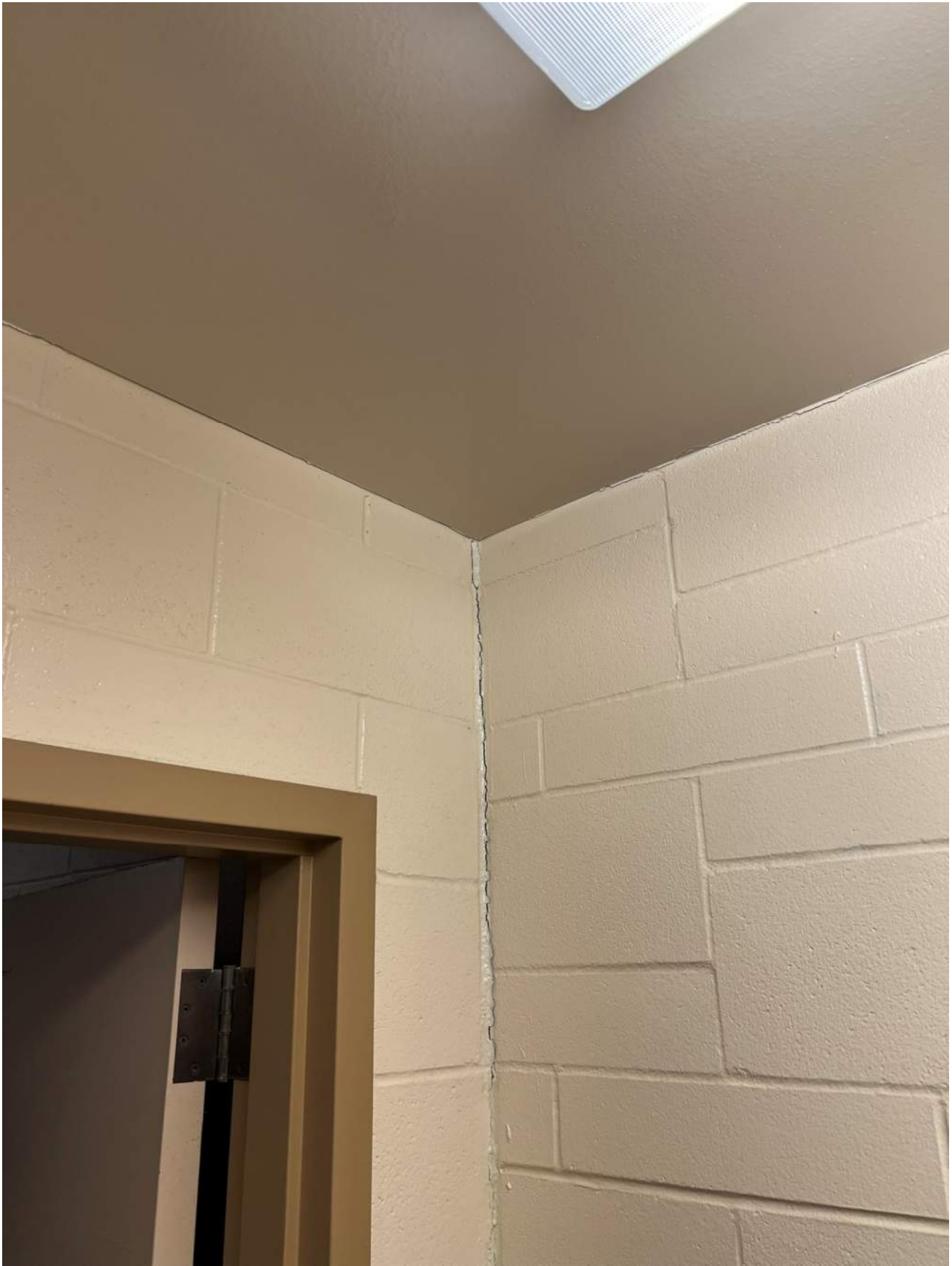
(Above: Cracks in wall of restrooms)
