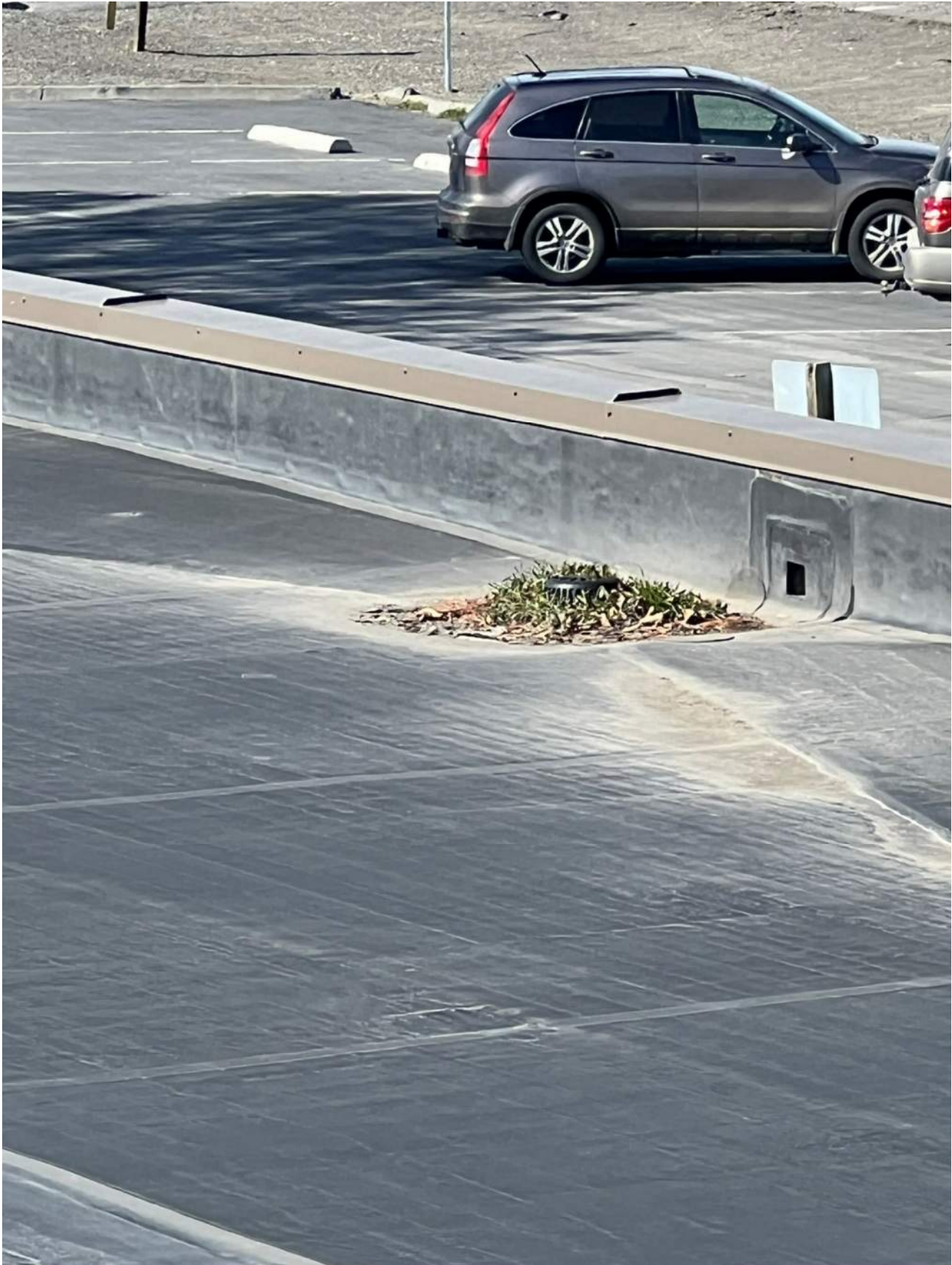
(Above: Roof debris and grass clogging drain)
