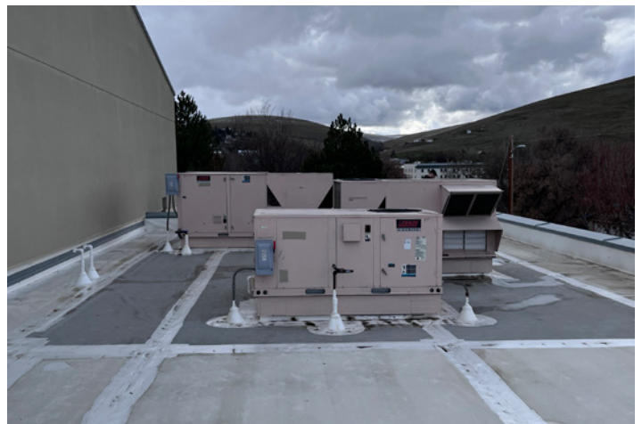
Roof and rooftop unit
