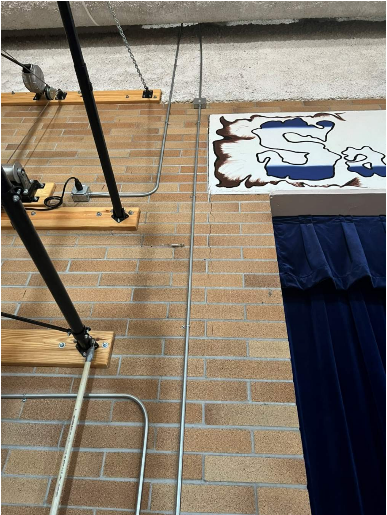
(Above: Minor cracks in pilaster adjacent to stage opening)
