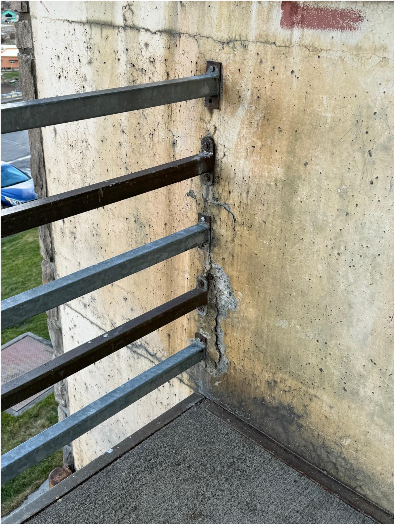
(Above: damaged guard rail connection)
