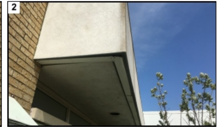
Replace metal soffit trim and wood blocking, typical. Repair cracks in plaster veneer.
