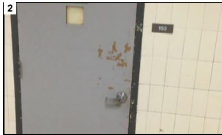
2 Fine Arts - Replace aged doors and frame.
