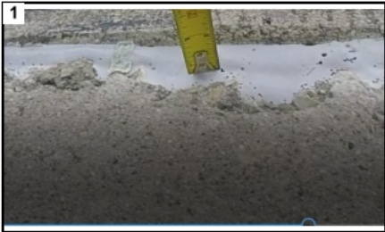
Greater than 1/2" vertical level change on path of travel.
