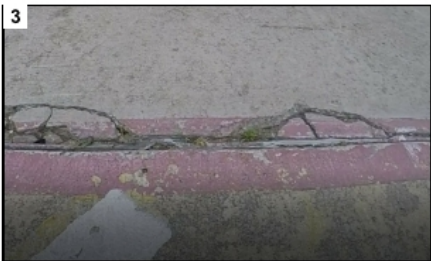
Broken pavement creates multiple level change violations along path of travel.
