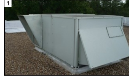
1 Trane rooftop a/c unit
