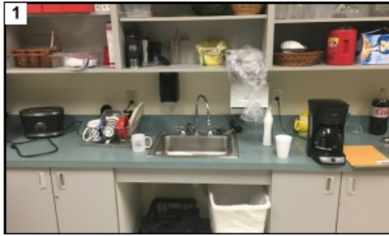
1 Admin - Replace aged casework in lounge.
