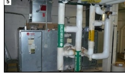
5 Lower level Trane VAV air handling unit
