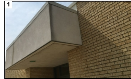
Replace metal soffit trim and wood blocking, typical. Acid wash plaster and masonry veneer.
