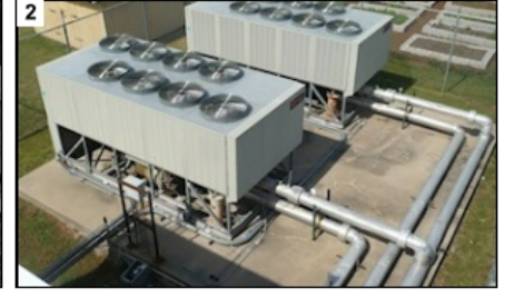
2 Trane air cooled chillers
