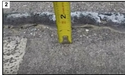
Greater than 1/2" vertical level change on path of travel. (3/4")
