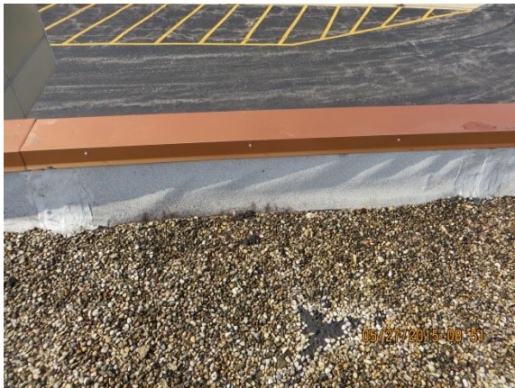
Photo 16: S Wall Blister By Vestibule Roof Drain
