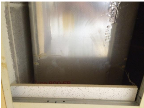
Photo 13: Room 118 Duct Insulation Stain
