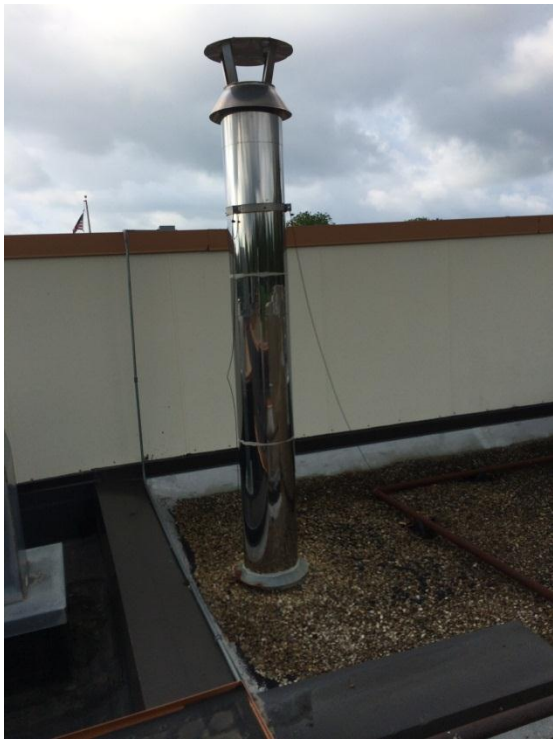
Photo 20: Unsupported Boiler Stack
