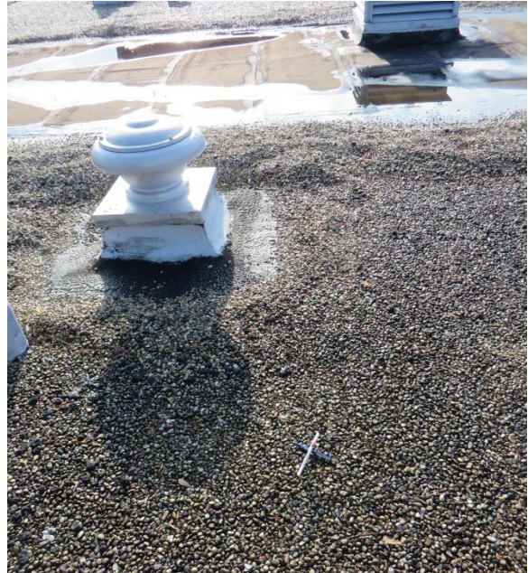
Photo 19: Soft Area By Office Exhaust Fan
