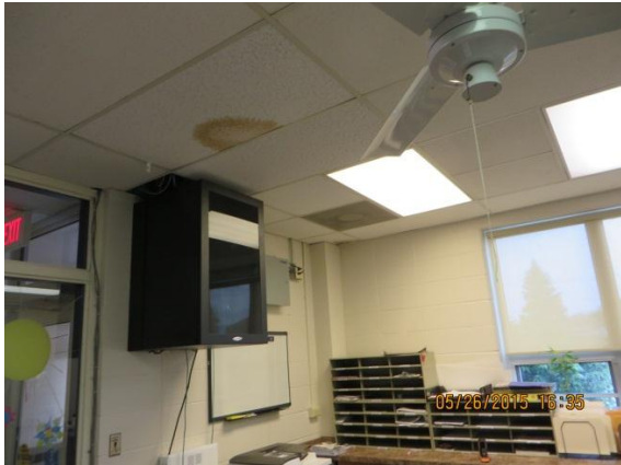
Photo 9: Stain by Technology Rack
