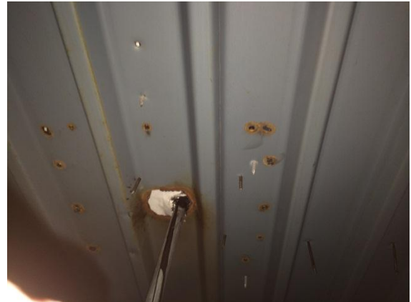
Photo 10: Conduit Above The Ceiling Stain
