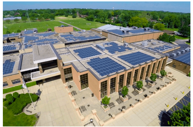
Lake Park HS Solar Installation Example
