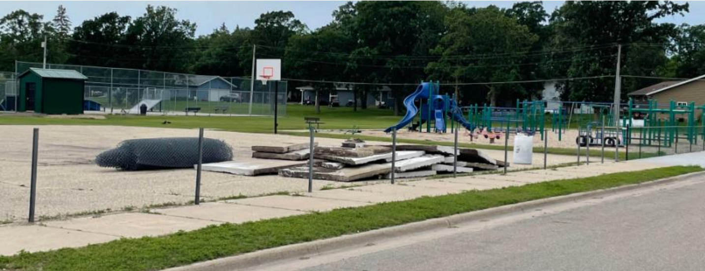
Old Sidewalk and fence removal underway to match new sidewalk and fencing installed last summer. Funding Source: Parking Lot improvement project - Abatement Bond
