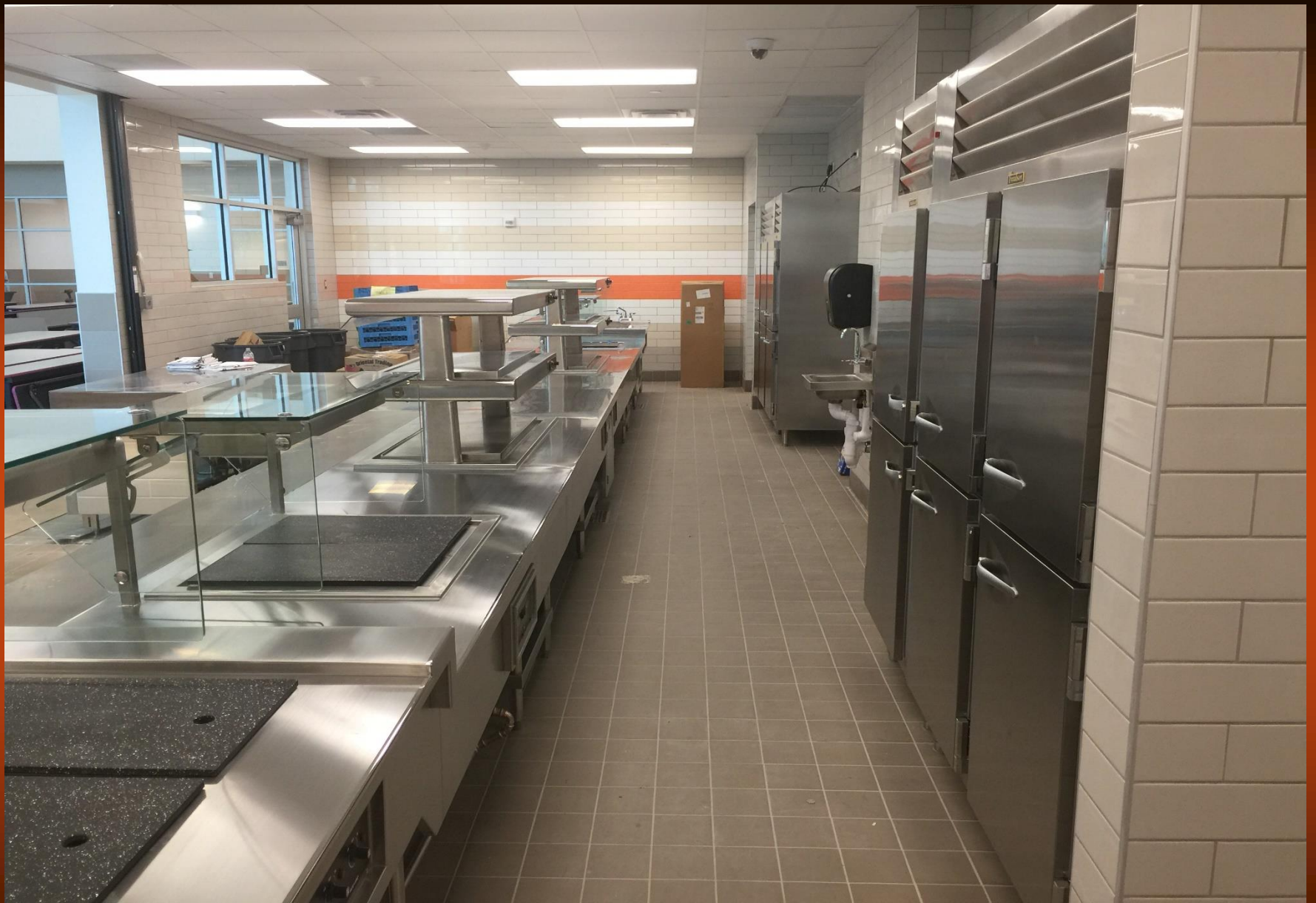
Walsh Elementary Kitchen Serving Line
