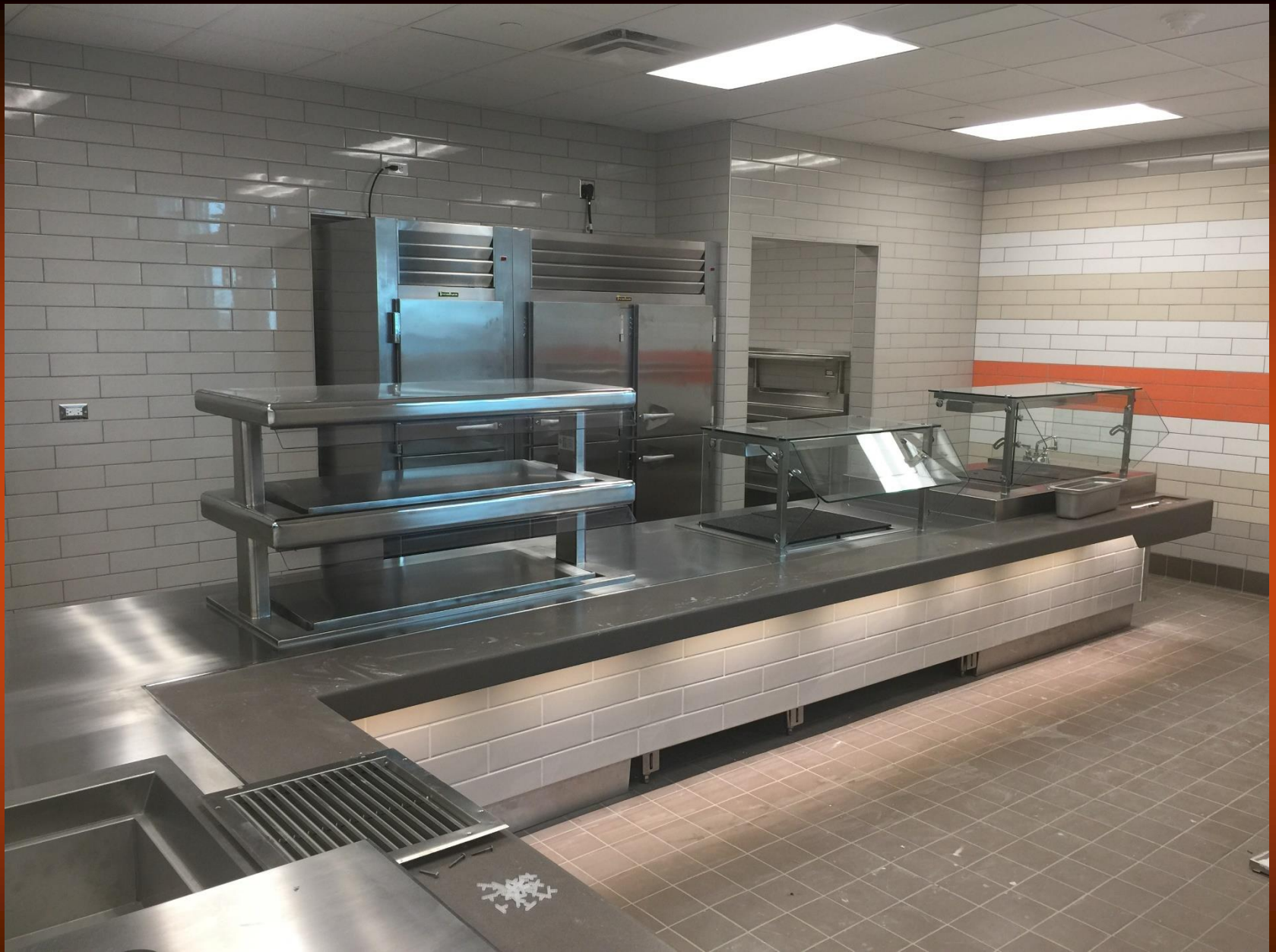
Walsh Elementary Kitchen Serving Line
