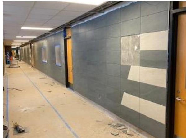
Figure 5 The wall outside the kitchen and extending down toward the locker rooms is well underway and currently still in progress.
