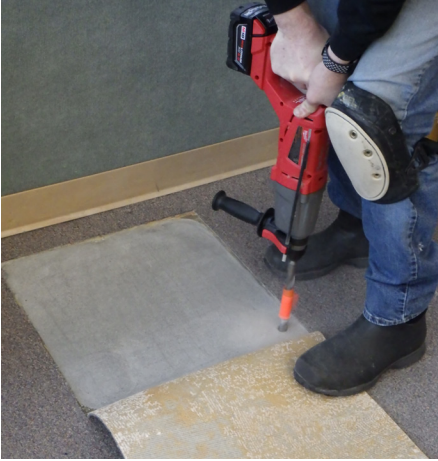
MRV and Dalhberg Design overseeing Rainbow Builders preparing slab for moisture vapor emissions and alkalinity tests. Testing results called for moisture mitigation measures for Riverbend Elementary in Juneau.
