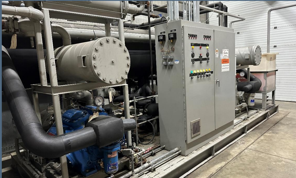
Aging Refrigeration System-Converted to RS-45 from R-22
