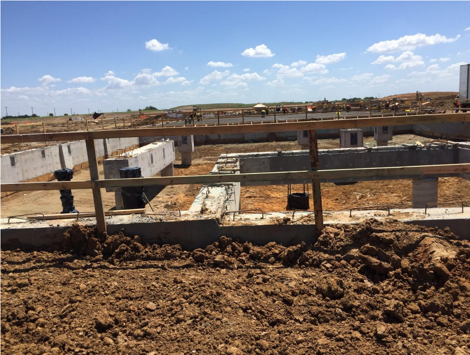
Area F Crawl Space and Area E Grade beams are under construction.
