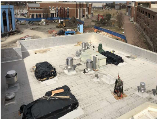
Exhaust Fans and Roof Curbs Installed at Kitchen Roof
