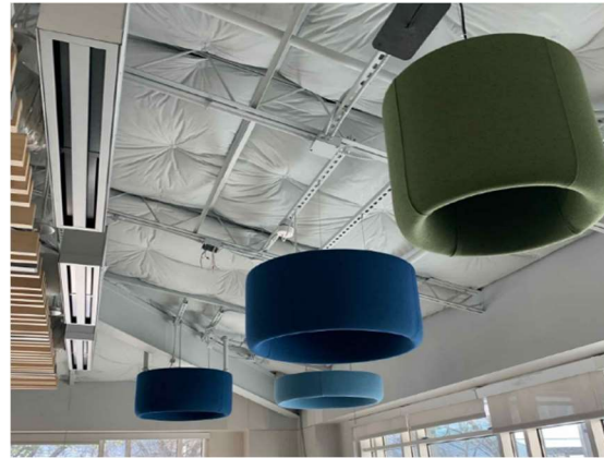
Decorative Lights Installed in Dining Hall at Alumni Hall
