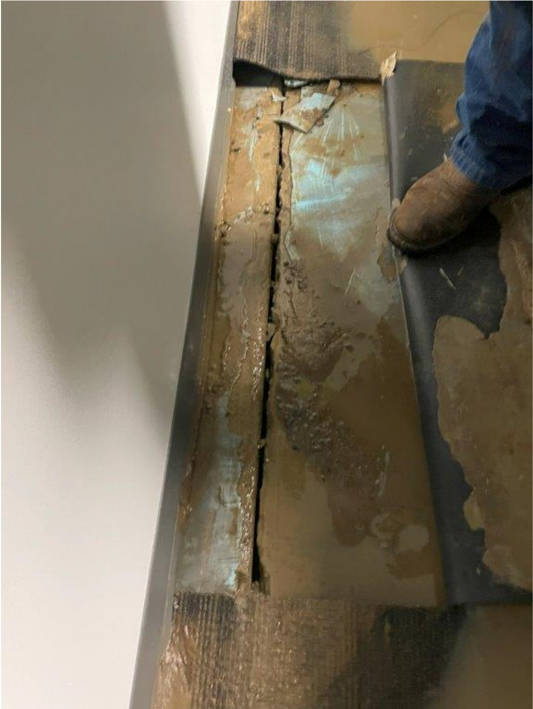
Photo 1: Infiltration Along Grade Beam and Slab
