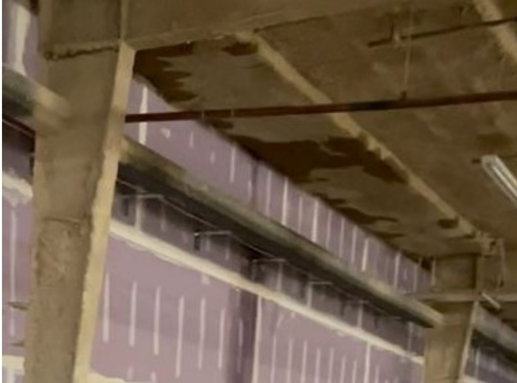
Photo 5: Water on west side of wall between the east and west wing, and indication of water on the underside of the roof in the west wing of the building.
