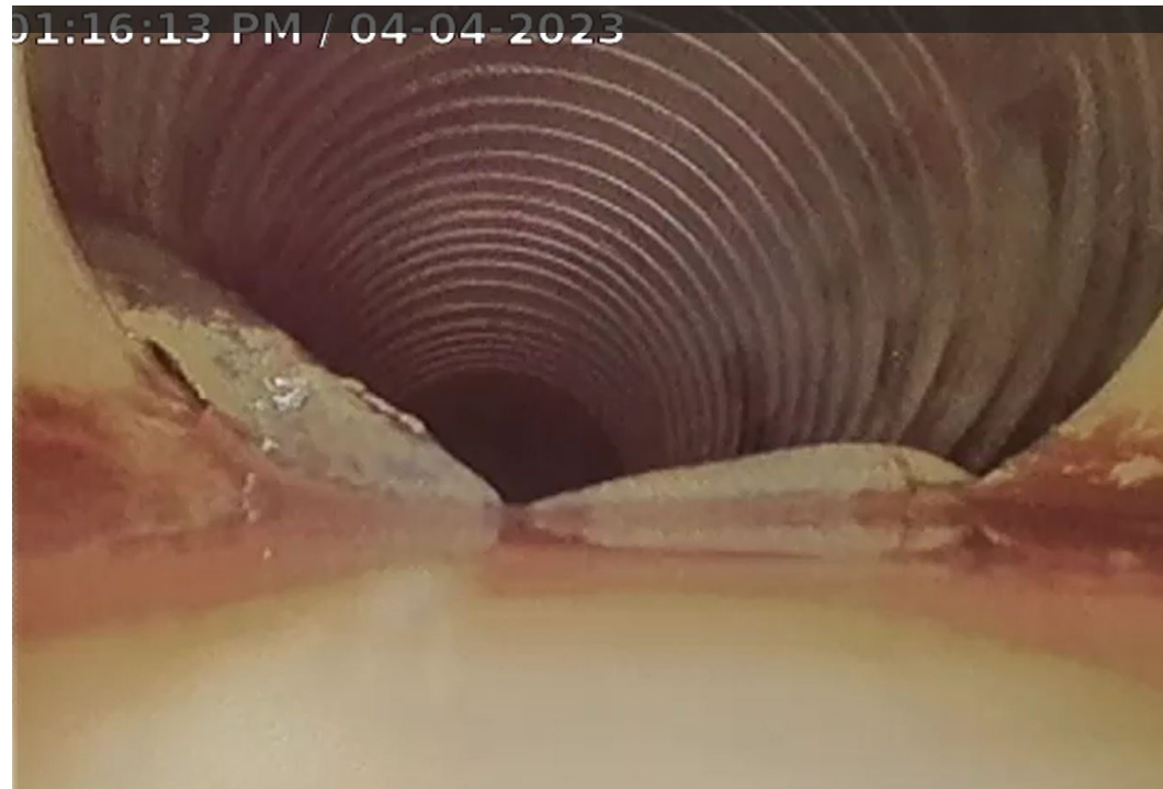
Photo 10: Poor connection of canopy roof 4-inch PVC to 4-inch corrugated piping.
