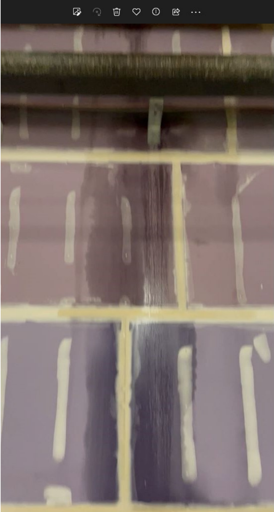
Photo 4: Sheet flow on wall between east and west wings of the building.
