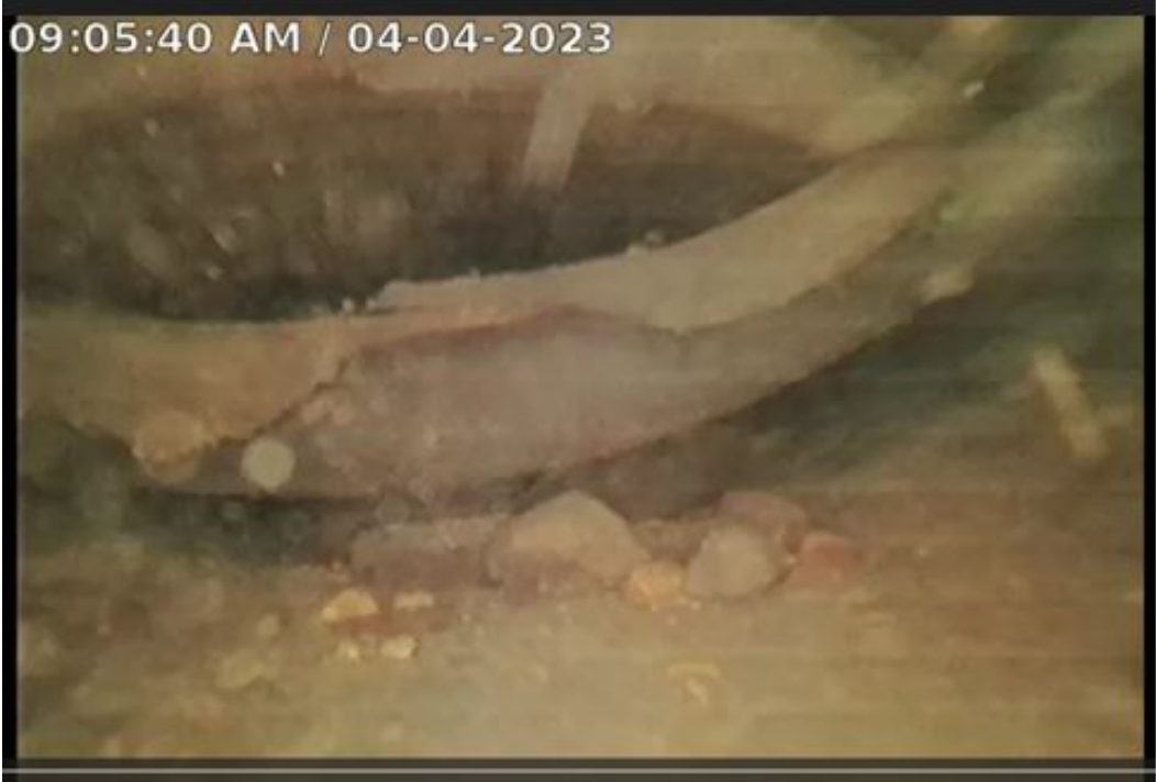
Photo 3: Piping Connection a Location 1.
