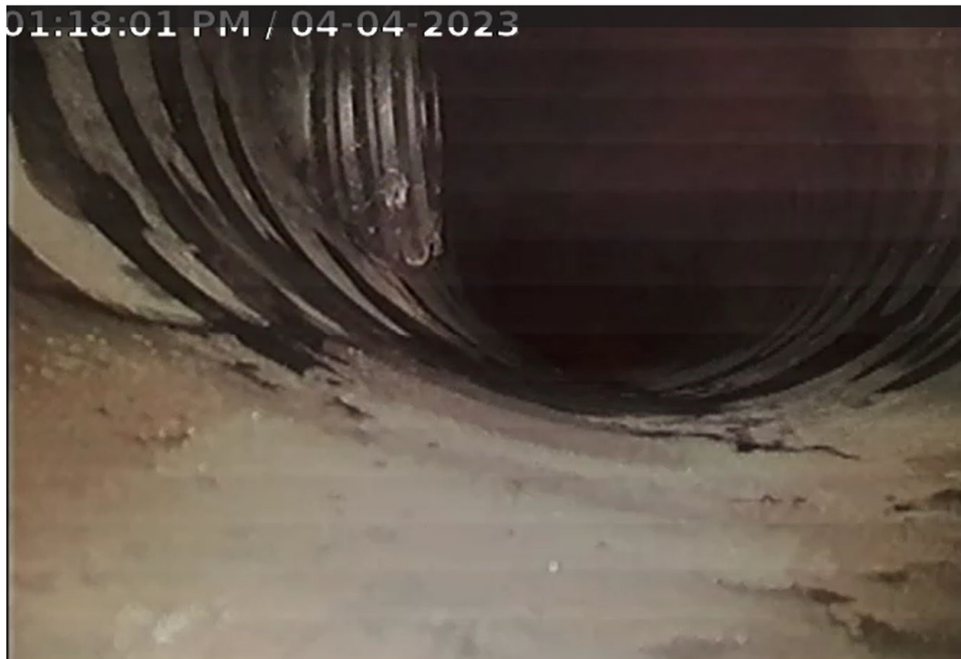
Photo 9: 4-inch corrugated penetrating through the wall of the 12 Inch corrugated pipe at Location 8.
