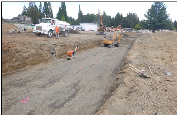
Stormwater detention system
