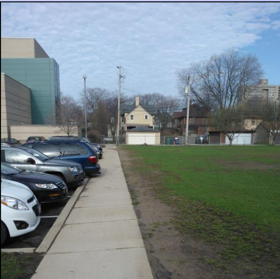
Typical eroded edge along sidewalk
