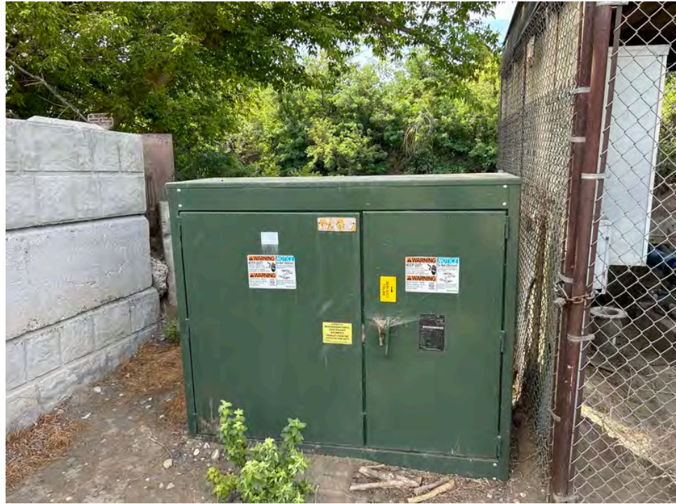
Photo 25. Pad-mounted transformer associated with irrigation pump
