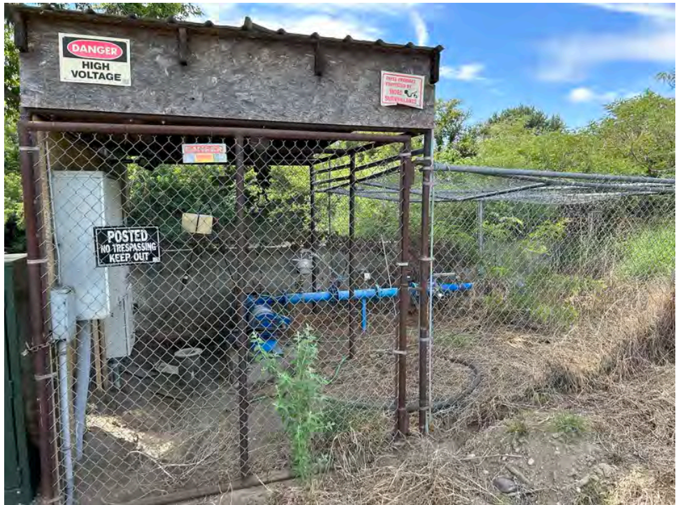
Photo 24. Irrigation pump located south of football field
