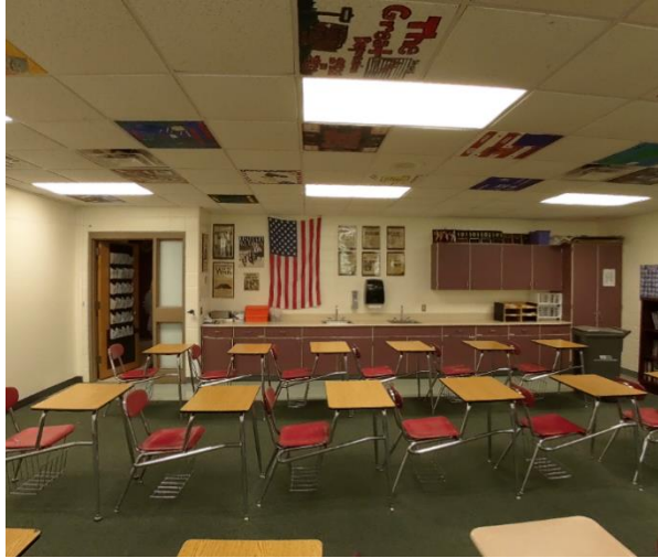
Outdated cabinets in classrooms.
