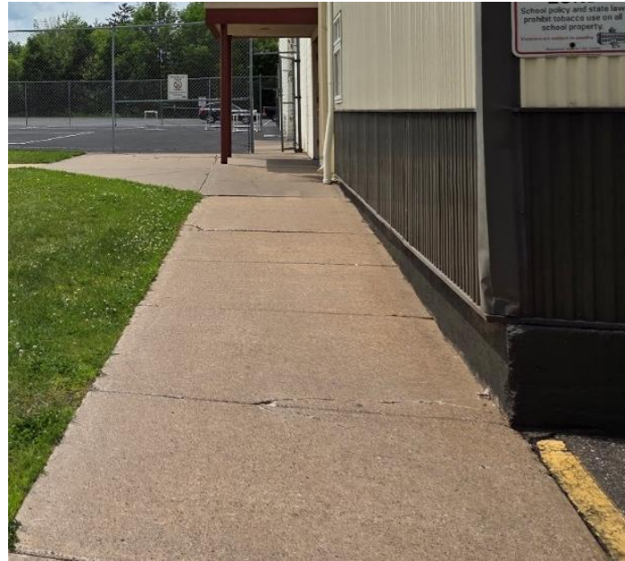
Cracks/wear found in the sidewalk next to the south part of the building.
