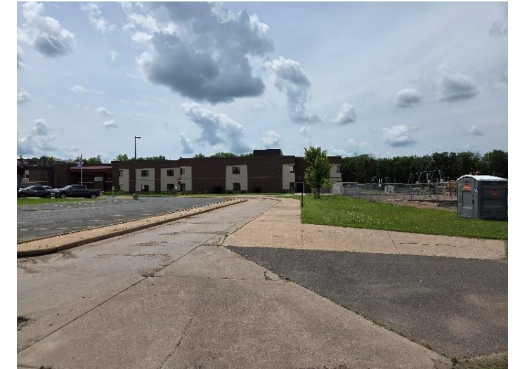
Cracks/wear found in the sidewalk and road by the east side of the building.
