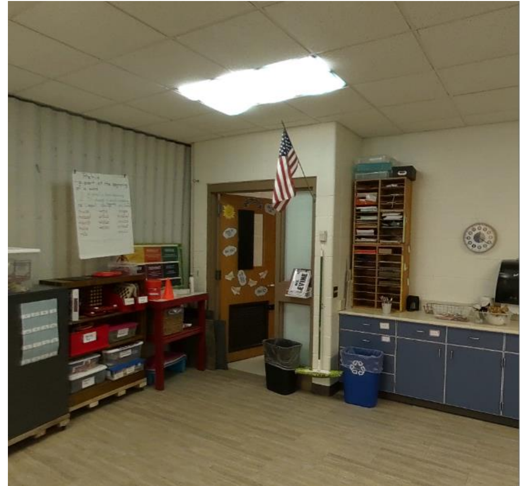
Vent on door in classroom.
