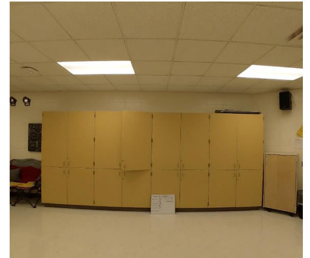
Outdated cabinets in choir room.
