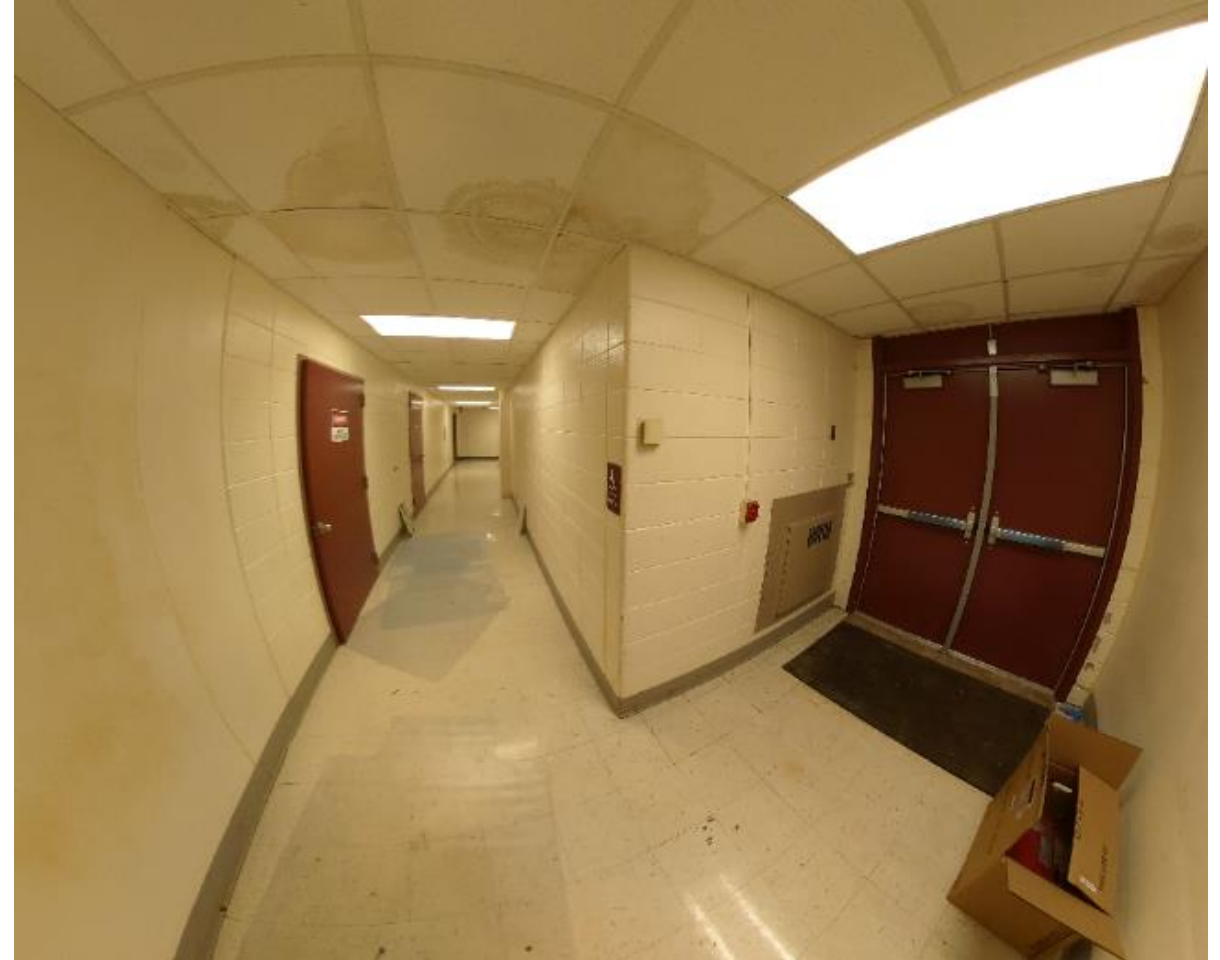
Aged ceiling tile with dark staining found in the 1962 section of the school.
