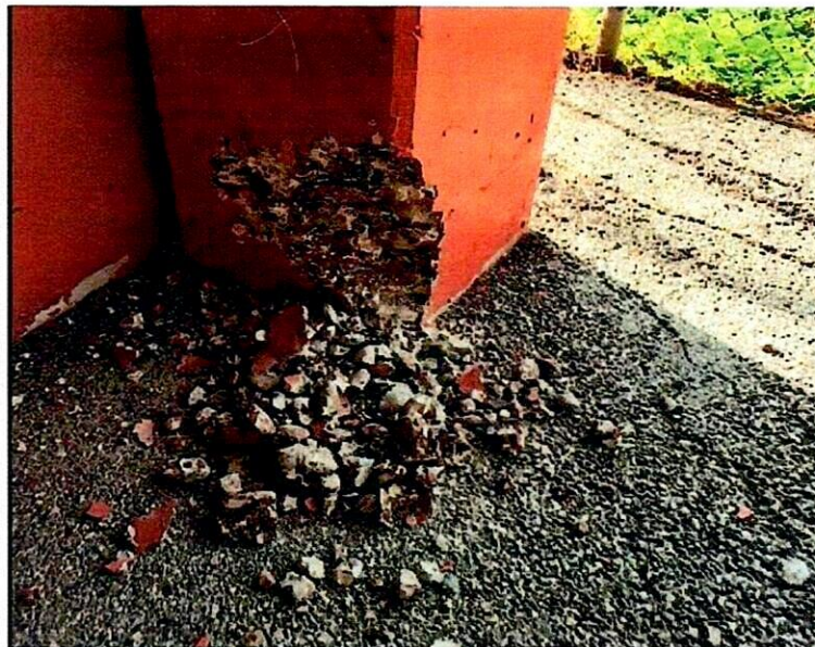
Photo #2: Column is Experiencing Spalled Concrete.
