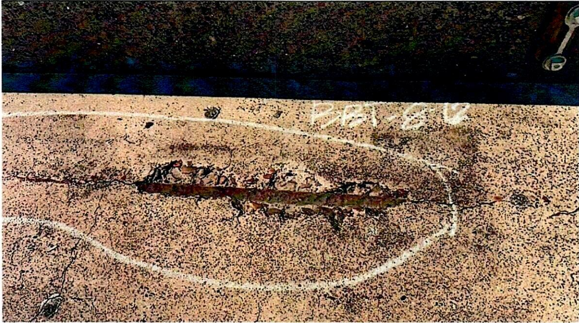
Photo 11: Bleacher Beam Topside Showing Exposed Rebar.
