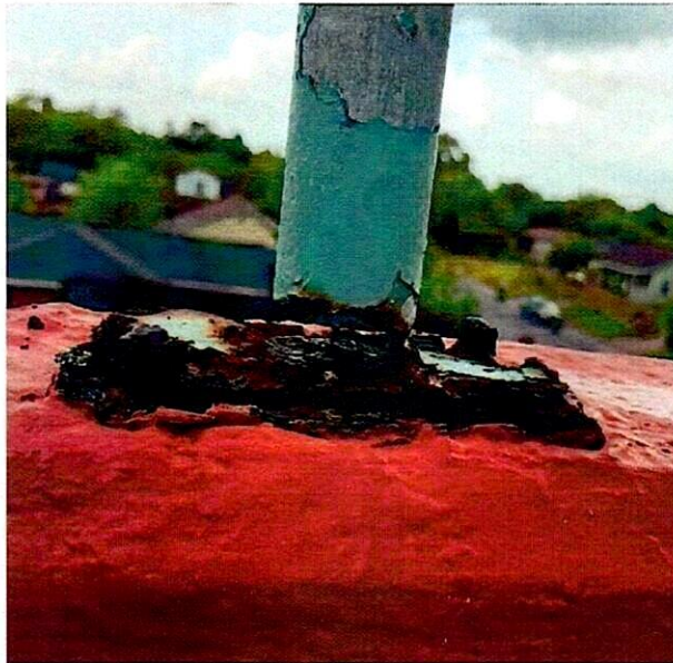
Photo 9: Guard Rail Base Plate Showing Severe Corrosion.
