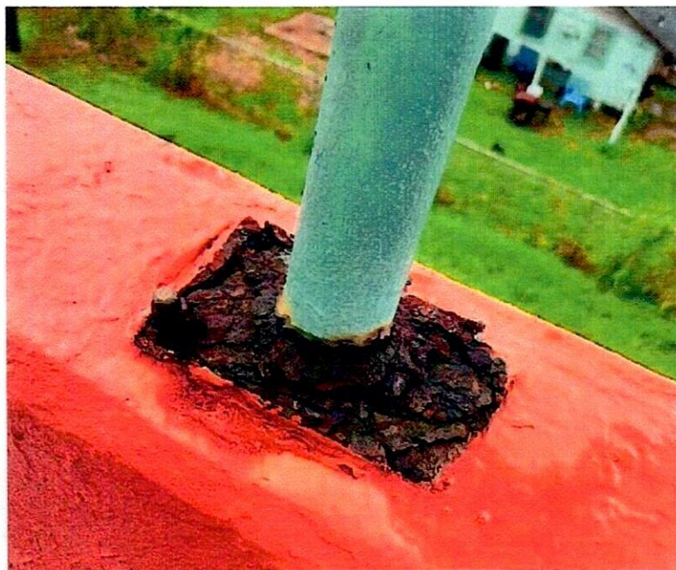
Photo 8: Guard Rail Base Plate showing Severe Corrosion.
