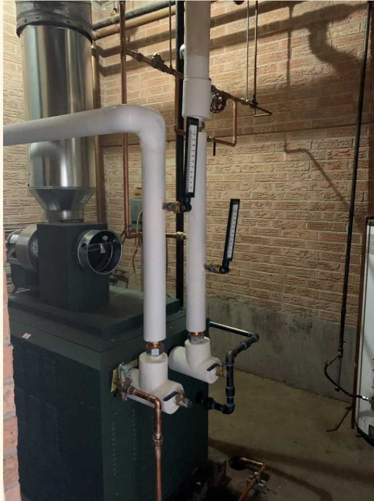
CDO Library Boiler
