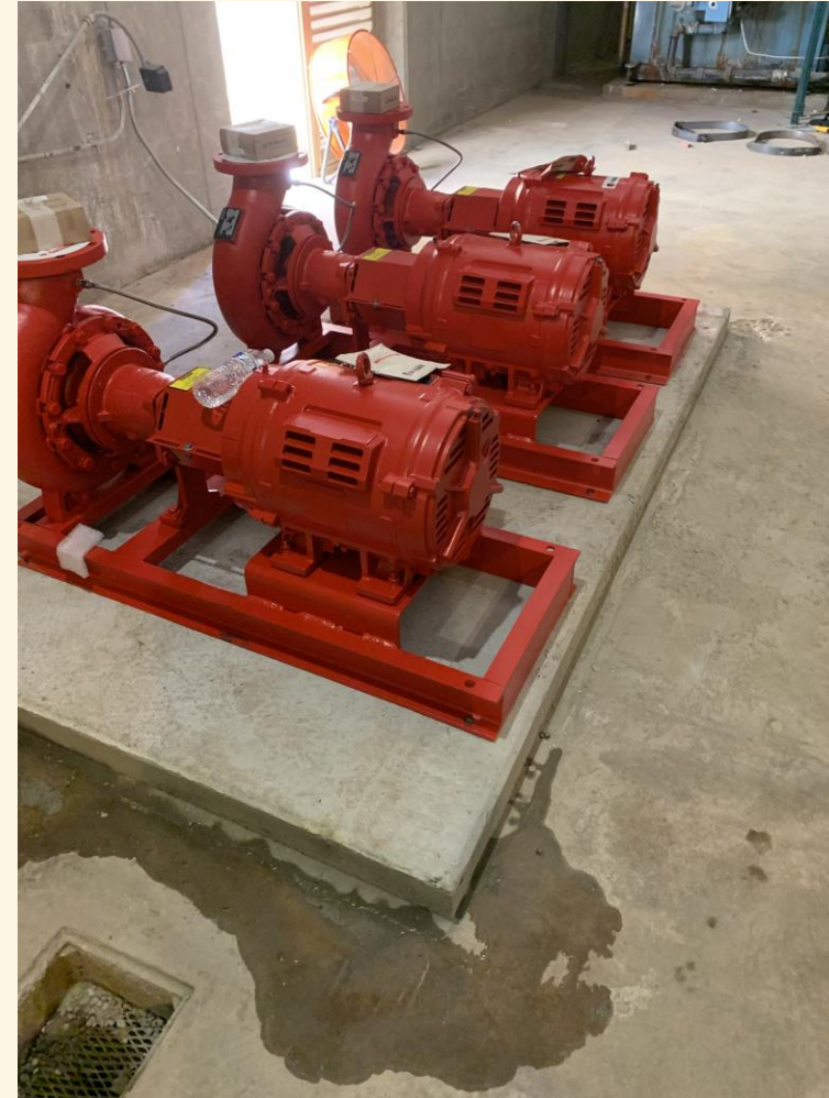
CDO Central Plant Pumps
