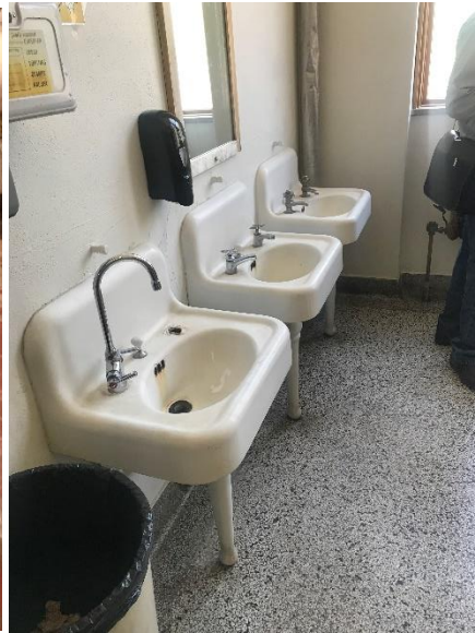
1920's PLUMBING FIXTURES
