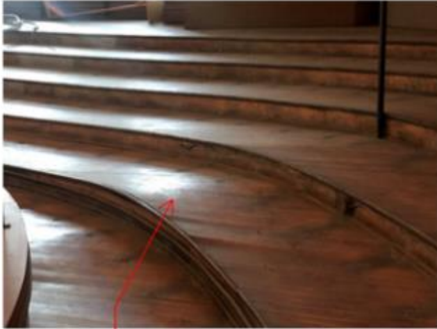
Water damaged wood floor at balcony
