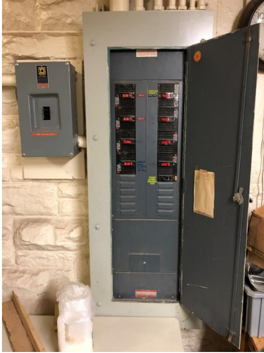
GENERAL ELECTRIC BOILER PANEL
