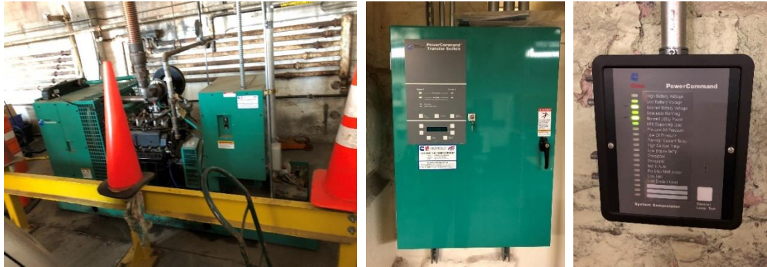
GENERATOR AND TRANSFER SWITCH
