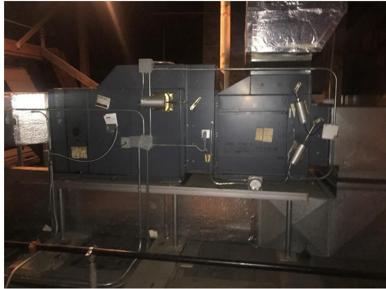
PNEUMATIC DAMPER ACTUATION
