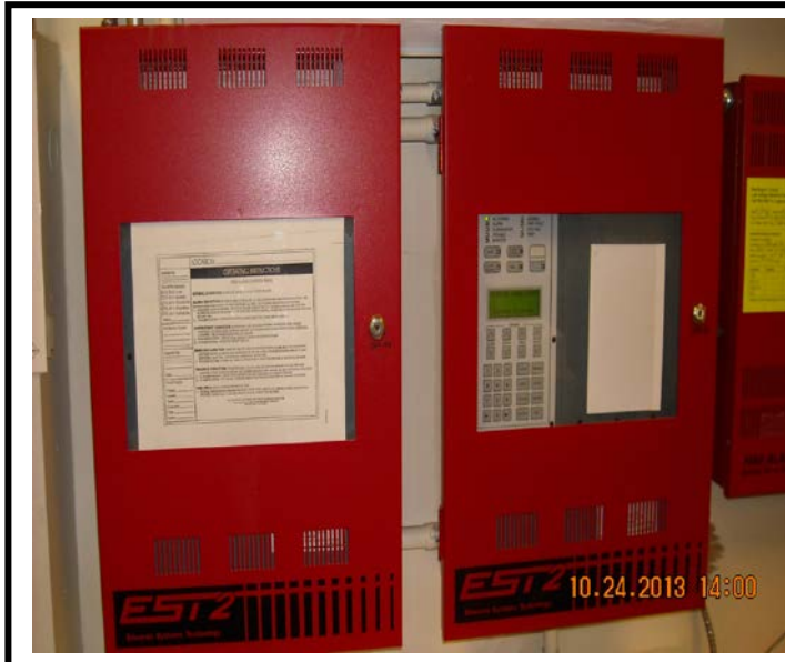
Fire Alarm Panel with Obsolete Technology
