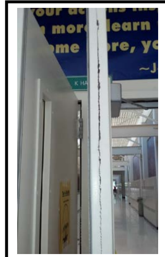
Door Separation Failure
