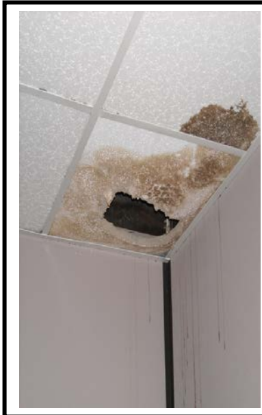
Roof Leak Damaged Ceiling
