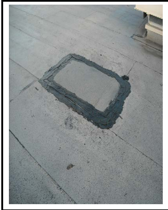
Example of a Patched Roof
