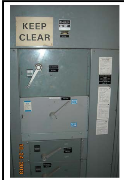
Obsolete Electrical Disconnect Panel
