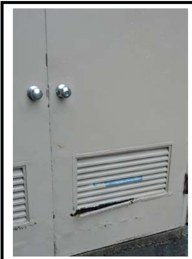
Damaged Grill & Rusted Door Panel
