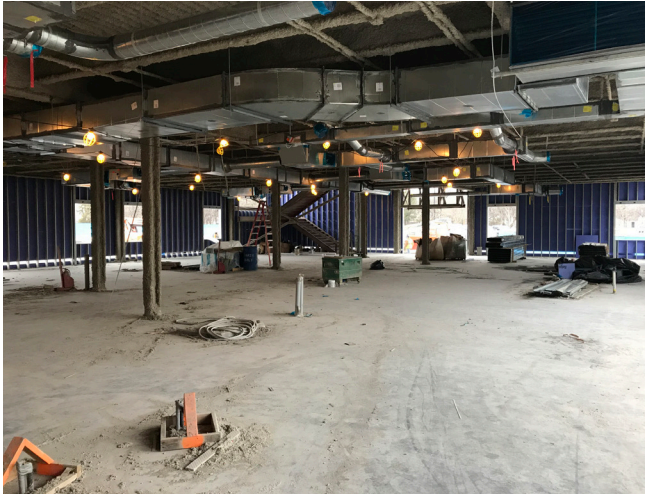
Area C - Overhead MEP
