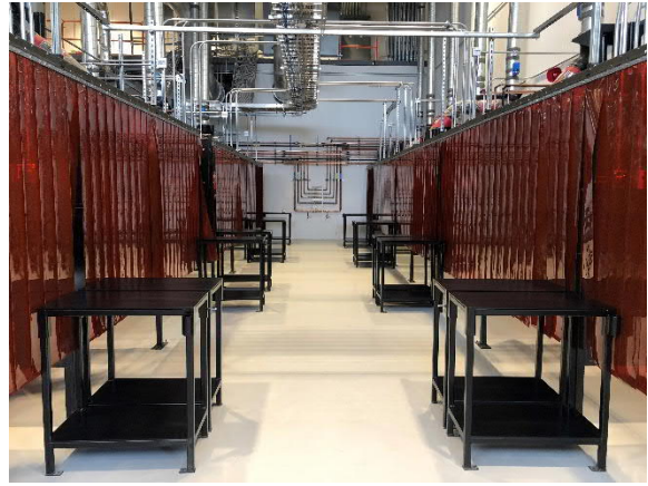
Welding Booths at Trade Bar B
