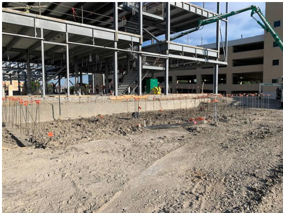
Utility Yard Area
