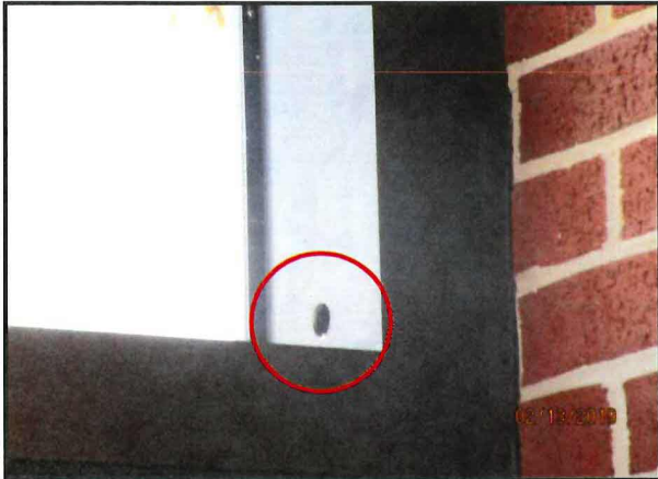
7. HOLE IN CURTAIN WALL FRAME
