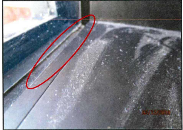
8. MISALIGNED INTERIOR GLAZING GASKET
