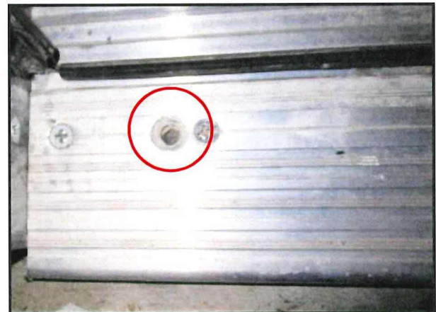
16. MISSING FASTENER IN DOOR THRESHOLD
