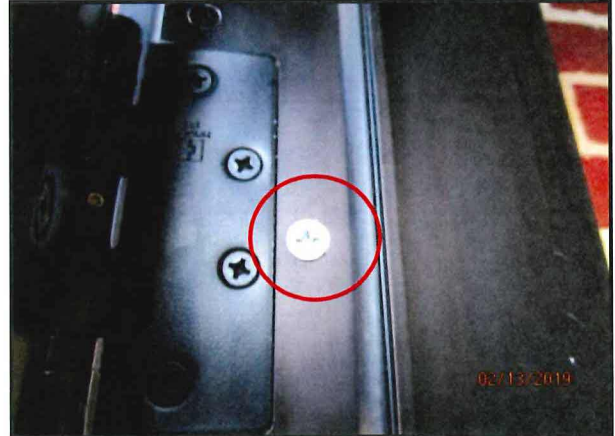
2. FASTENER HEAD FINISH DOES NOT MATCH ADJACENT FRAMING
