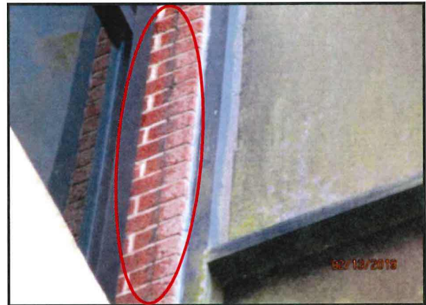
4. REMNANTS OF SEALANT ON SURFACE OF EXTERIOR BRICK VENEER
