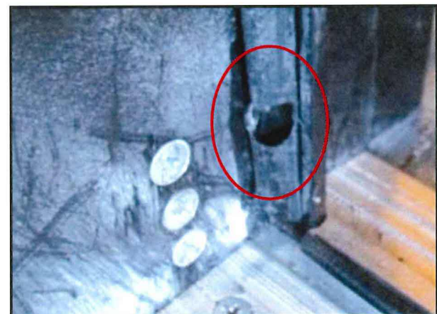
24. DAMAGED WEATHERSTRIPPING ON DOOR
