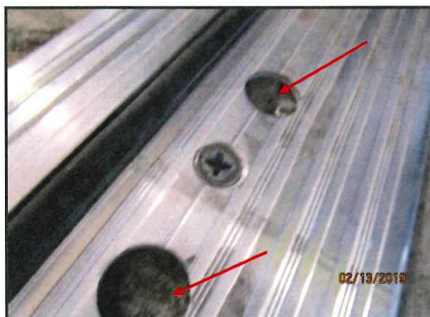
17. CONCRETE NOT DRILLED OUT AT DOOR PANIC ROD INSERT LOCATIONS
