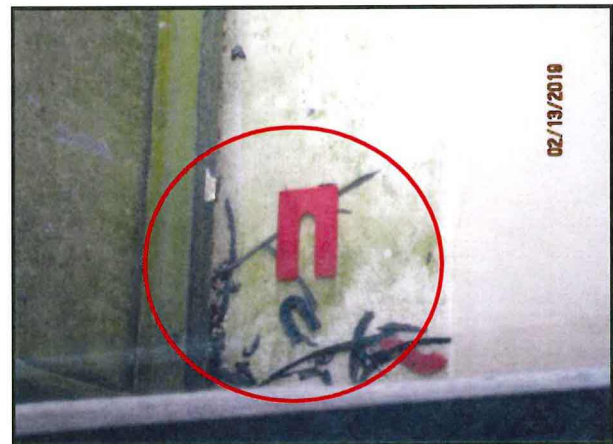
12. DEBRIS ON EXTERIOR WINDOW LEDGE AT LEVEL 2
