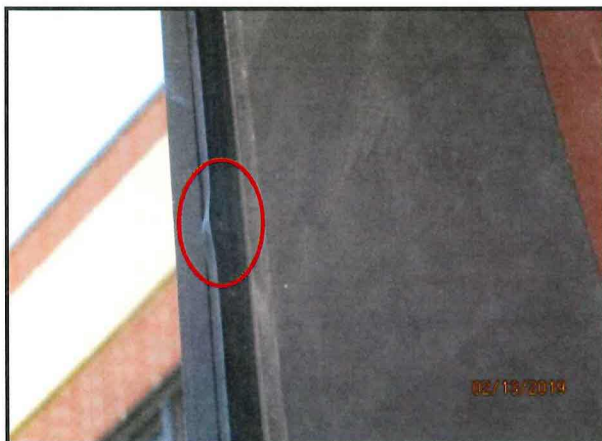
15. DISINGAGED EXTERIOR GLAZING GASKET
