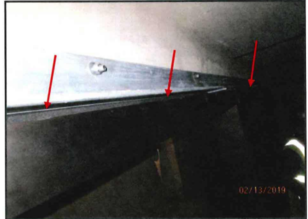
14. MISSING SEALANT AT TOP OF WINDOW AT INTERIOR
