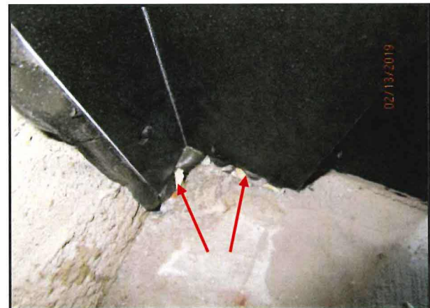
22. INADEQUATE SEALANT AT BOTTOM OF SHEET METAL CLOSURE
