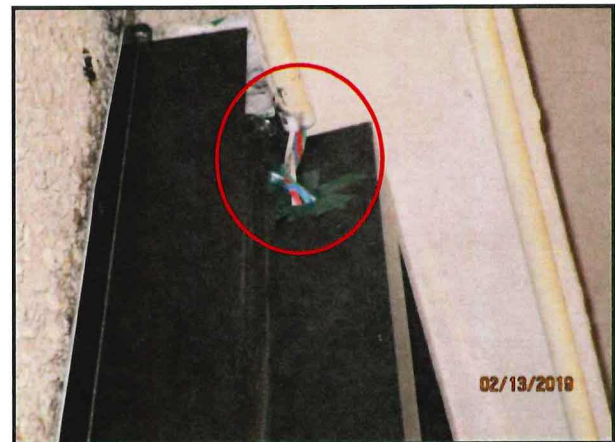
6. UNPROTECTED ELECTRICAL WIRES (wiring not encased within conduit or closure)
