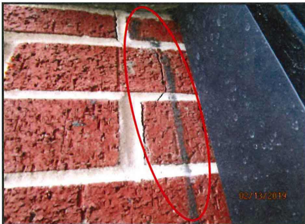
3. REMNANTS OF SEALANT ON SURFACE OF EXTERIOR BRICK VENEER
