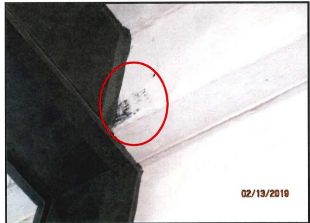
10. STAIN ON INTERIOR WALL
