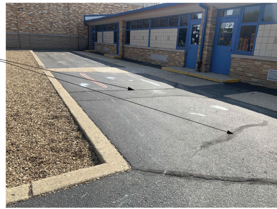
POWER WASH FULL EXISTING AREA OF WORK AND CRACKFILL ALL DAMAGED OR CRACKED ASPHALT LOCATIONS WITH ACRYLIC CRACKFILLER, TYPICAL
