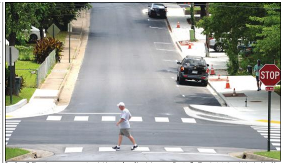
People walk Thursday near a new section of sidewalk along Church Avenue in Fayetteville. The city is in the middle of a $3 million project using bond money that voters approved in April 2019 to install new streetlights and sidewalks in the city's downtown. (NWA Democrat-Gazette/Andy Shippe)
