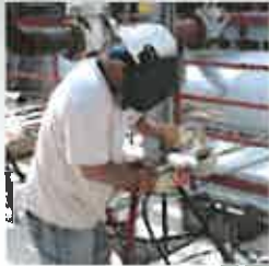
INDUSTRIAL PROCESS PIPING
