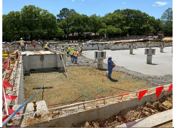
Fig 6: Mud Slab Area D
