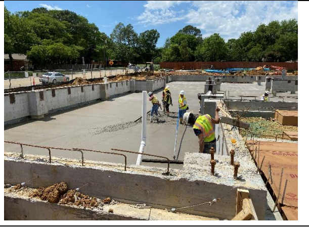
Fig 8: Mud Slab Area D
