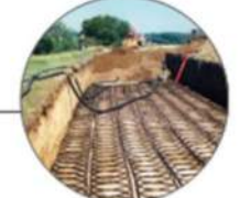
GEOTHERMAL WELL FIELDS
