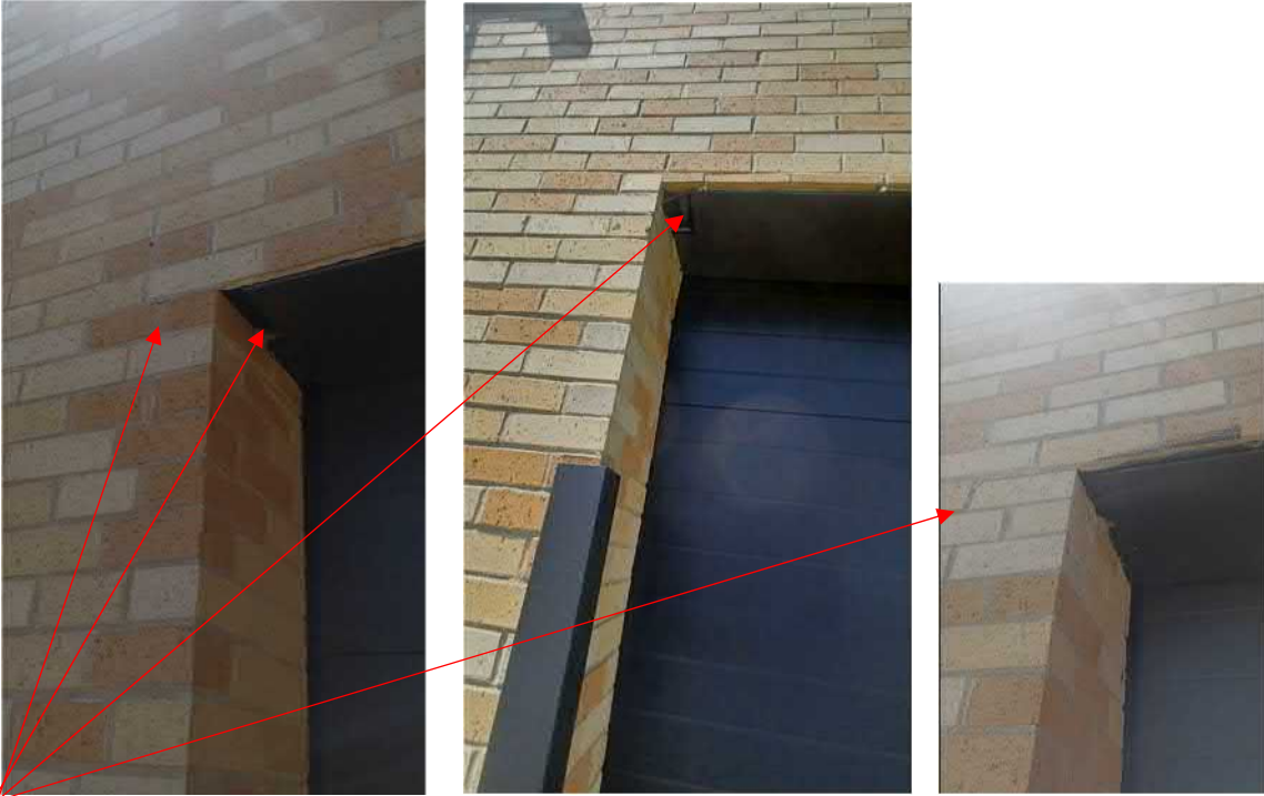
Figure 5: Some cracking mortar and bricks at bearing ends of lintels. Brick ledge/plate several inches short of wall @ over head doors.
