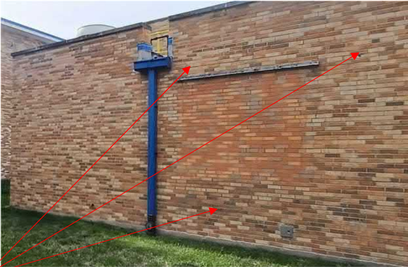
Figure 9: Area of brick in need of tuckpointing. Broken brick in need of replacement. Cast stone 'intel' in need of power washing and joints tuck pointed and sealed. note: Stone parapet caps (above) will be capped in metal when roofing is replaced in the future.
