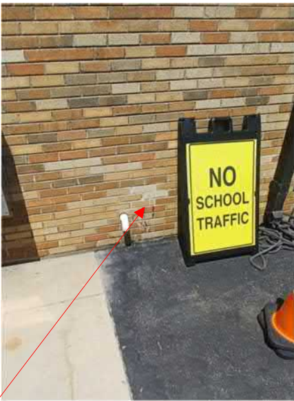
Figure 6: Small area of brick needing tuckpointing and cleaning.
