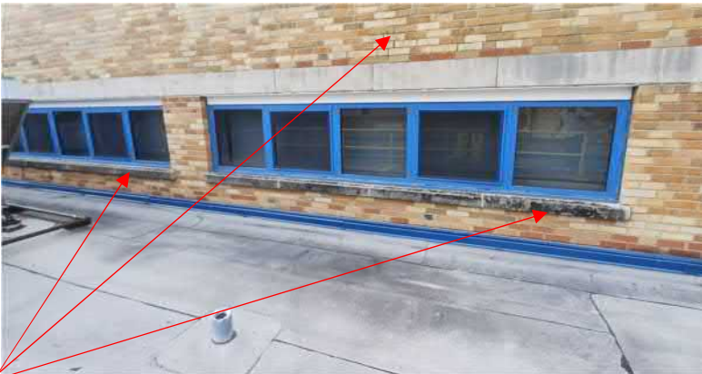
Figure 10: Areas of brick and cast stone sills (around roof #10, and in the courtyard) in need of tuckpointing, power washing and sealing.
