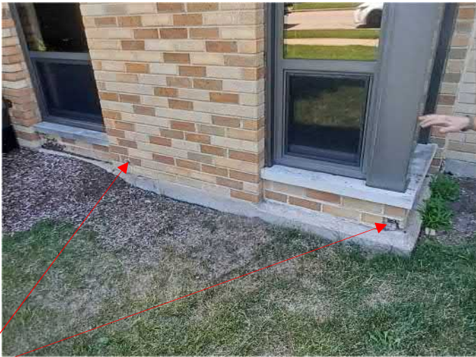
Figure 4: Some broken bricks and mortar joints in need of repair. Cast stone sills, in need of power washing and re-pointing and sealing of joints.
