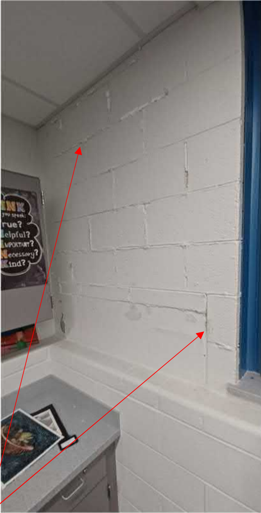
Figure 8: Water damage evident at interior CMU, in classroom @ bottom of brick pier.
