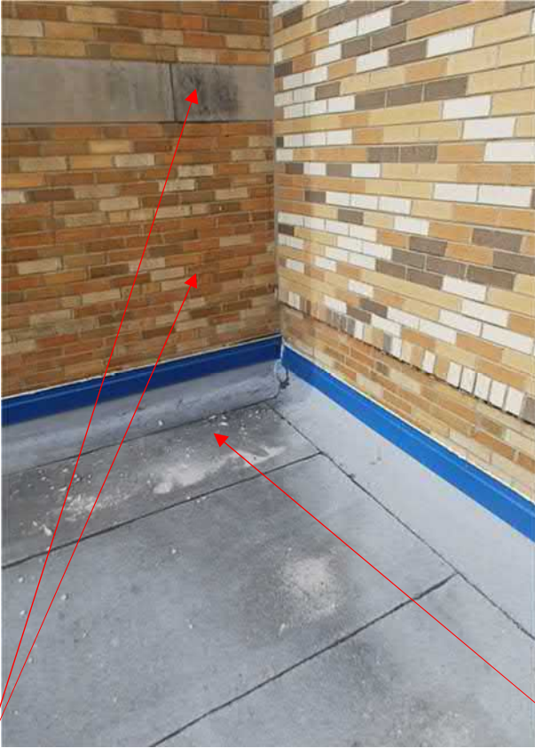
Figure 11: Areas of brick and cast stone sills (around roof #10, and in the courtyard) in need of tuckpointing, power washing and sealing. pieces of mortar on the roof deck.
