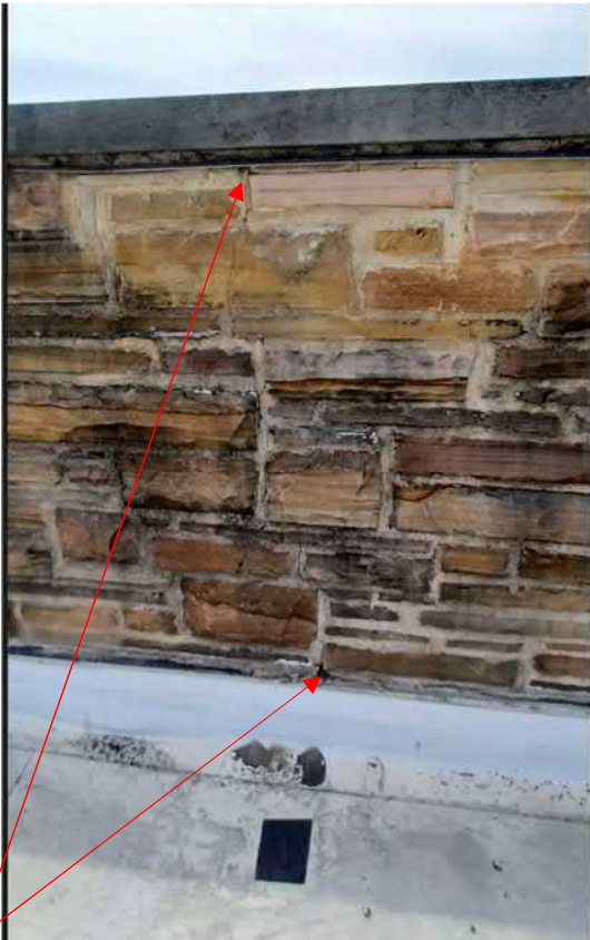
Figure 15: Areas of cracked and broken limestone in need of repair, tuckpointing and cleaning.
