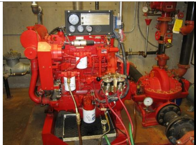
SEISDTBS Diesel operated fire suppression pressure booster pump. In good condition.
