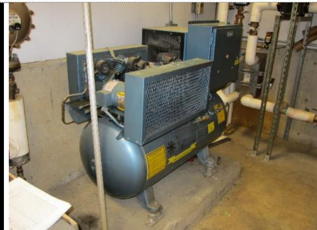
SEISDTBS Air compressor used to keep dry fire sprinkler charged.
