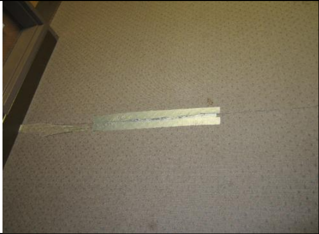
SEISDTBS Worn out carpet. New carpet is already on site. Replacement is due over Christmas break. Project was listed as priority 5 on CIP list.
