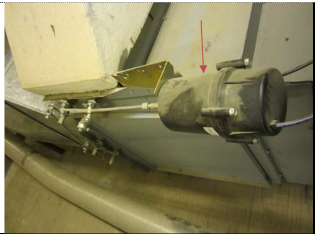
SEISDTBS Some of these pneumatic parts have not been manufactured in years. Upon failure, it has become nearly impossible to find original replacements.
