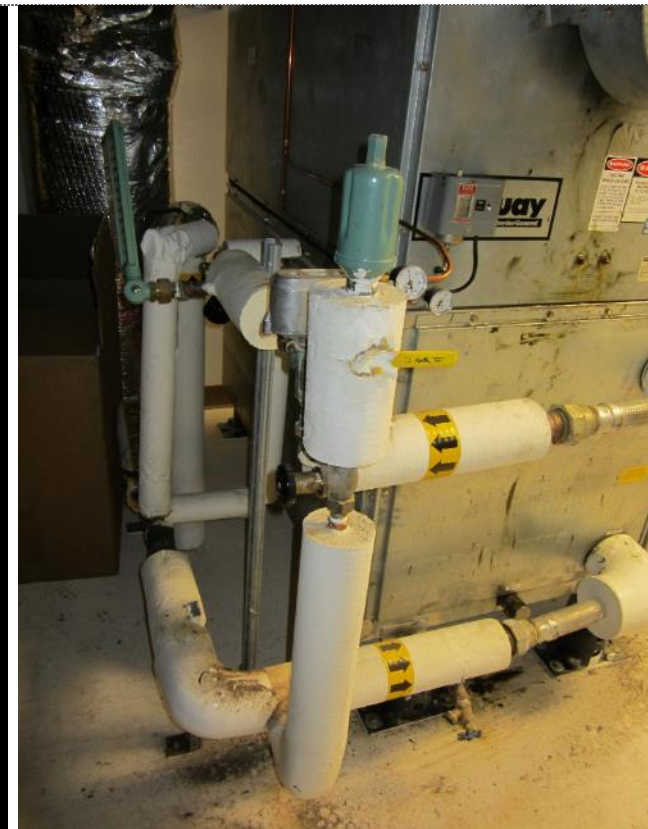
SEISDTBS HVAC automation in gymnasium is marginally achieved via defective pneumatic controls. Maintenance personnel need to manually interact with systems as on-demand / as-required basis.
