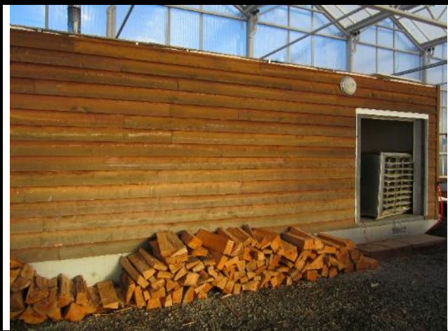
SEISDCCGH Boiler unit located inside of greenhouse.
