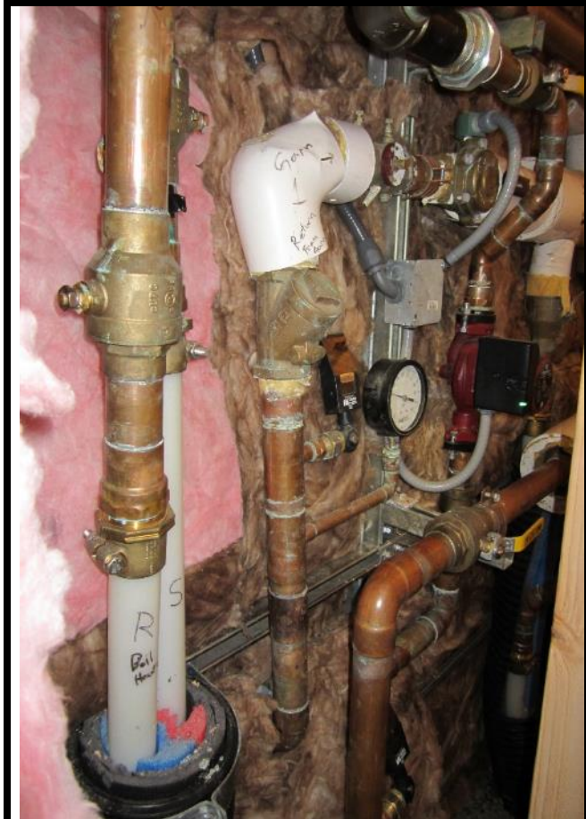
SEISDTBSBBF Distribution system - polyethylene glycol- behind the boilers. Very basic and effective.
