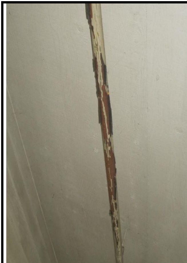
SEISDTBS Failing fire sprinkler piping –dry system. Replacement is priority 1 on CIP list.
