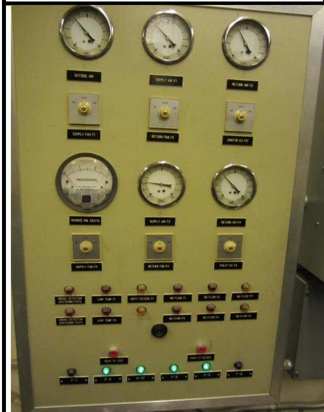
SEISDTBS HVAC control panel, main schools. Some of it appears to be functional.
