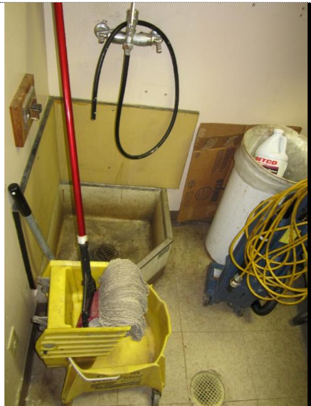
SEISDTBS Custodial closet. This part of the building is of original construction.
