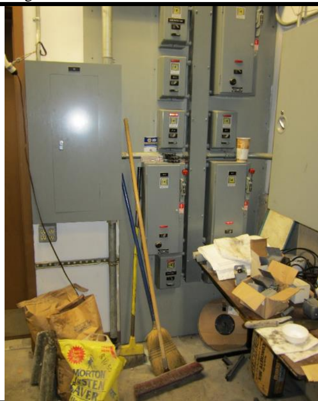
SEISDTBS Electric panels access - need 36" clearance in front of them.
