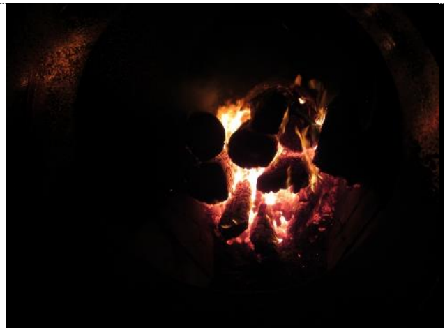
SEISDTBSBBF Inside combustion chamber. Boilers are opened to atmosphere (non-pressurized vessel) and therefore do not require state inspection. Operational caution must be exercised, however, not to produce internal heat exceeding boiling point.
