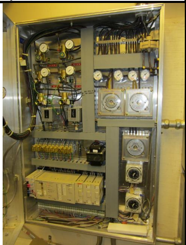
SEISDTBS Hybrid system, part pneumatic, part electronic. District plans to upgrade this antiquated system. Project is listed as priority 4 on the district's CIP list.
