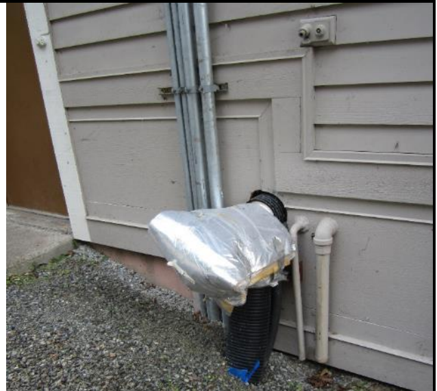
SEISDTBS Wall penetration for biomass boiler insulated piping into main facility.
