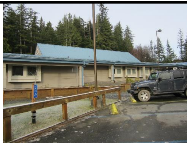
SEISDTBS Roof replacement is priority 2 on CIP list.
