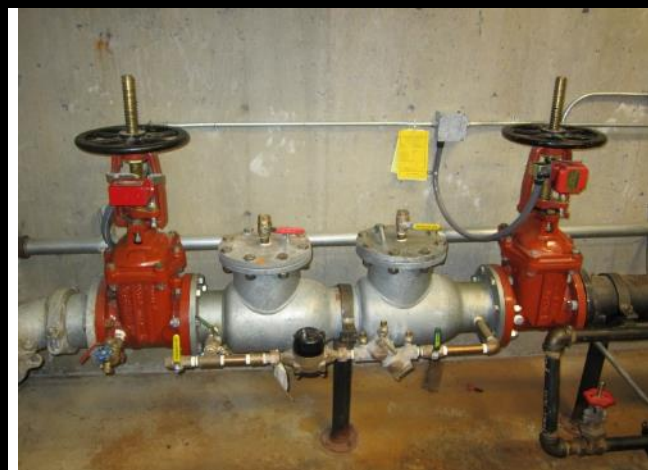
SEISDTBS Check valve. Inspection last completed in October 2015.
