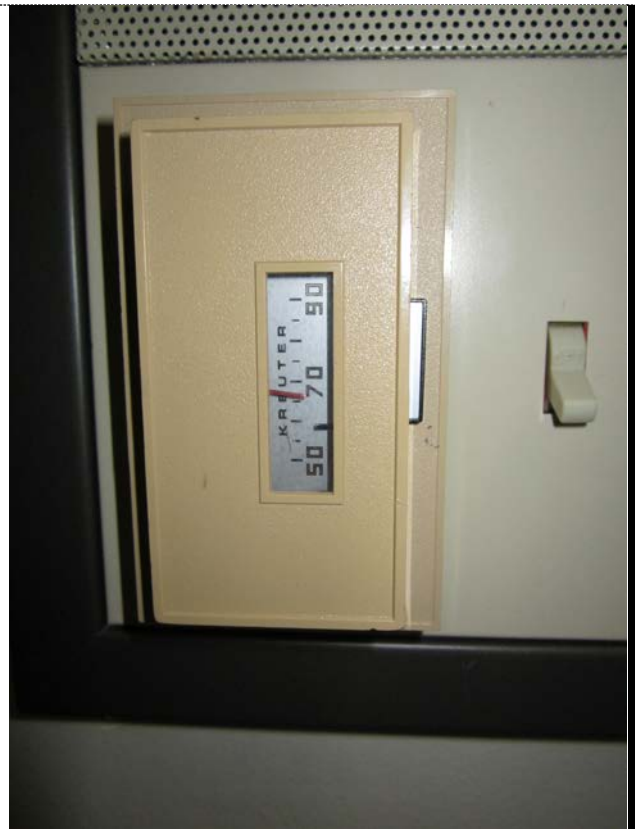
SEISDTBS Temperature reading of 66 degrees Fahrenheit. Site visit was conducted during in-service day (no students).
