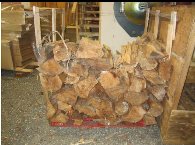
SEISDTBSBBF Wood ready to be burned. Boiler -1 of 2- in background.
