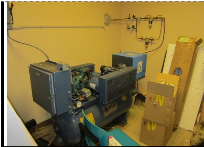
SEISDTBS Air compressor with strainer / dryer. Used for HVAC pneumatic controls.
