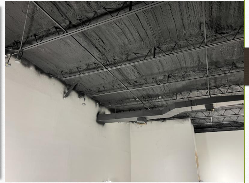
NOC Insulated Ceiling
