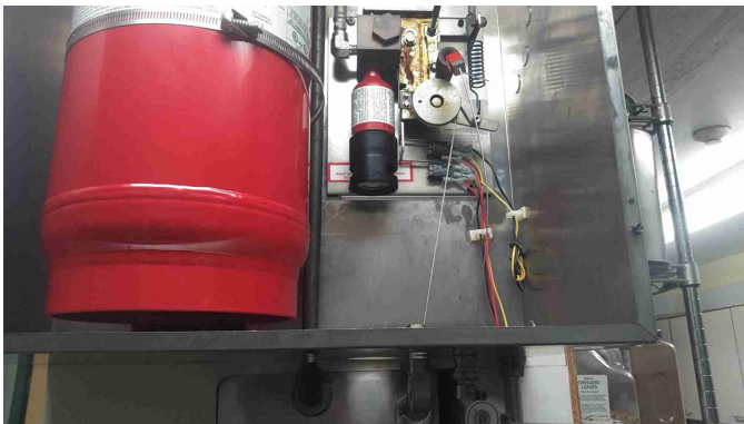
SYS #1 - Incorrect Detection Cable Installation
