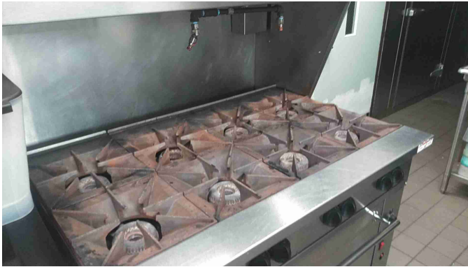
SYS #1 - Appliance Line/Old Nozzles and Locations
