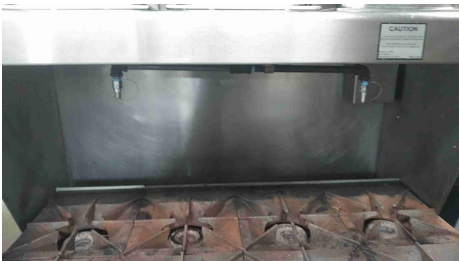
SYS #1 - New Nozzle and Piping Location
