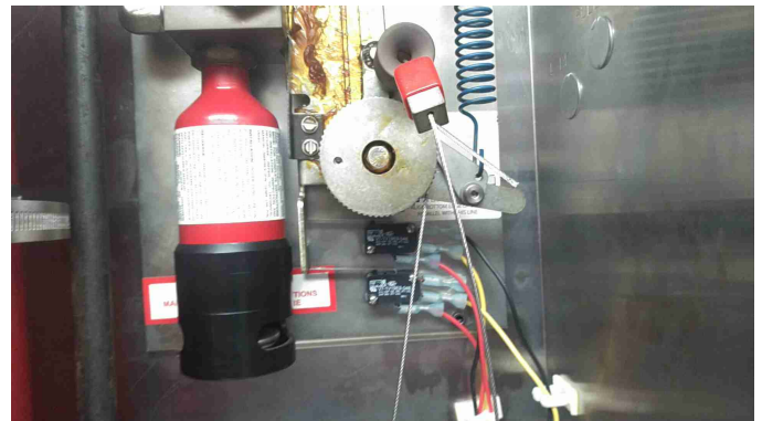
SYS #1 - Incorrect Detection Tension
