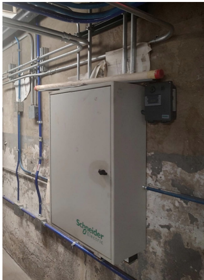
CO2 DETECTOR INSTALLED
