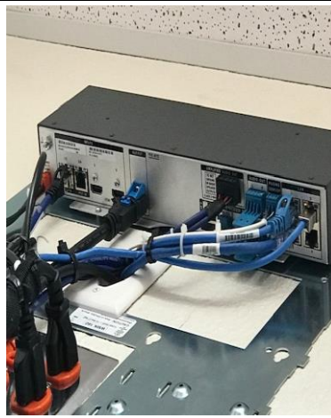
Closer look at the inside of the Wall Vault. The Wall Vault is the control station or the 'brains' of the Extron System.
