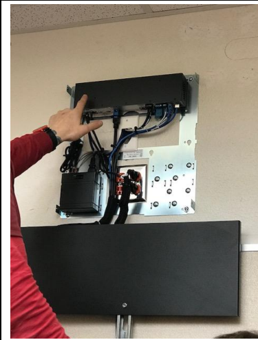
Inside of the Wall Vault. This holds the electrical, network and other cabling components for the system.
