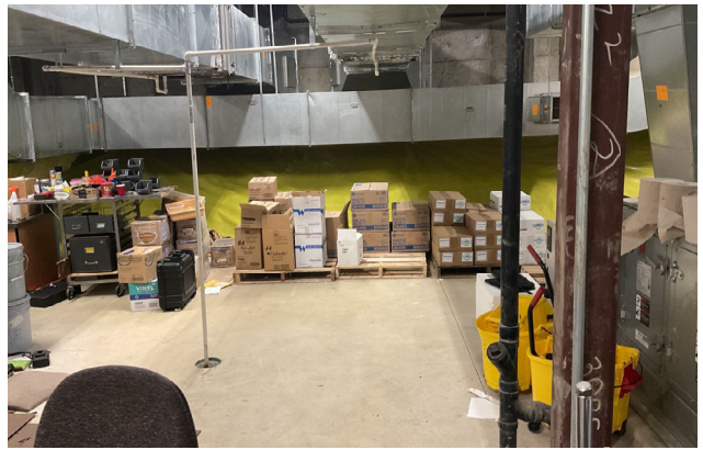
DLR Group image of NKN Middle School's unsprinklered mechanical room - which cannot exist as storage by code.
