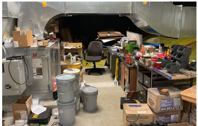
DLR Group image of NKN Middle School's unsprinklered mechanical room - which cannot exist as storage by code.
