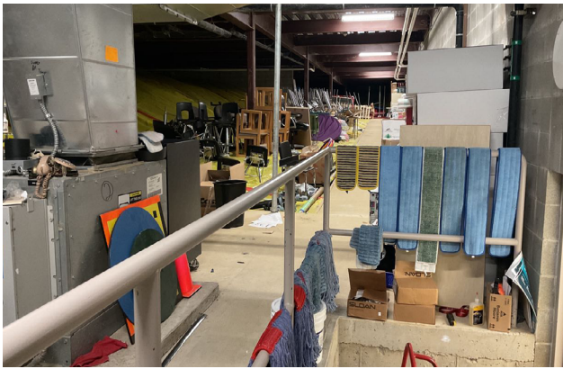
DLR Group image of NKN Middle School's unsprinklered mechanical room - which cannot exist as storage by code.
