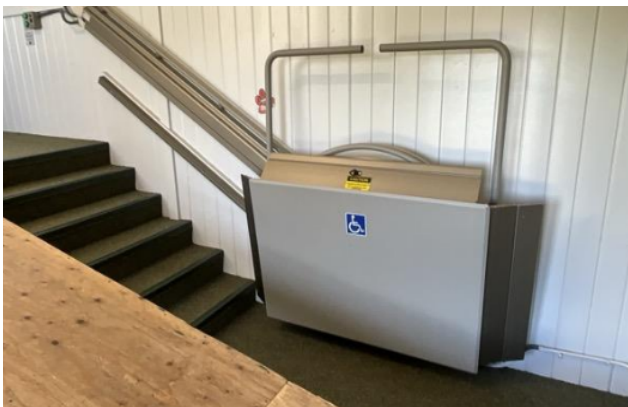
Bureau Veritas image of Garibaldi's centralized stair-climbing lift system, connecting to upper level classrooms.
