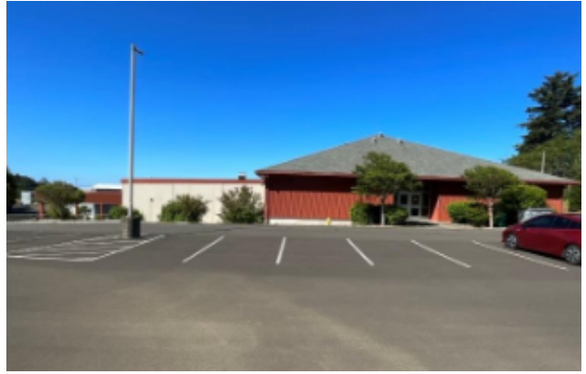
Bureau Veritas photo of "dark spot" caused by a lack of site lighting (also see pole barn, baseball fields, & back lot).
