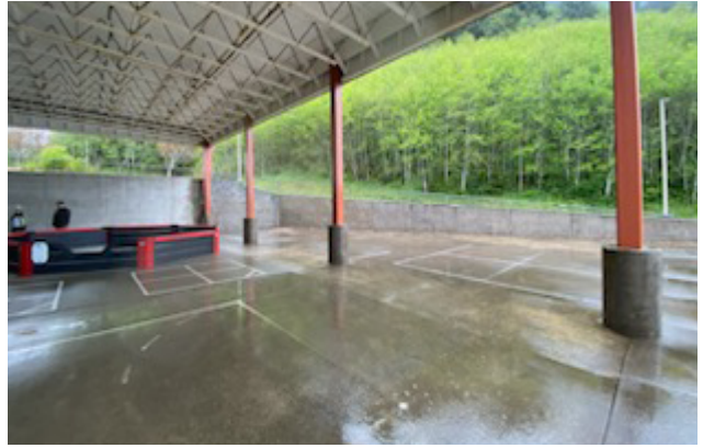
Bureau Veritas image of NKN Middle School's covered play area which is not fully enclosed/protected from elements.
