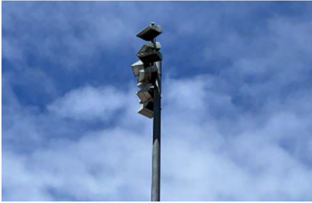
Bureau Veritas photo of NKN High School utilities - which have largely been piece-mealed from outdated systems.
