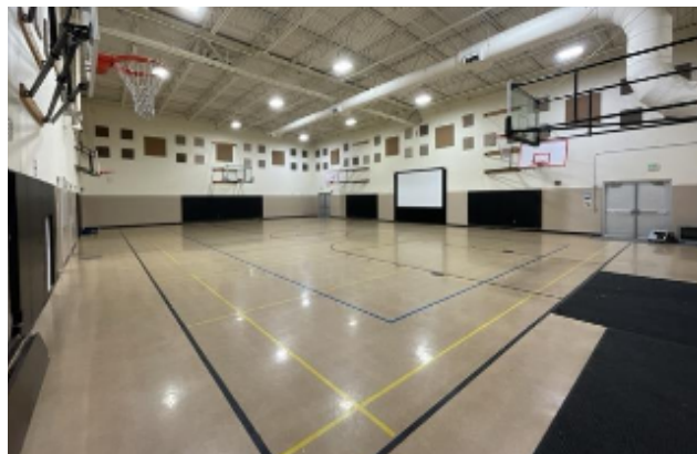
Bureau Veritas image of NKN Middle School's multipurpose gymnasium, which cannot support athletic teams/bleachers.
