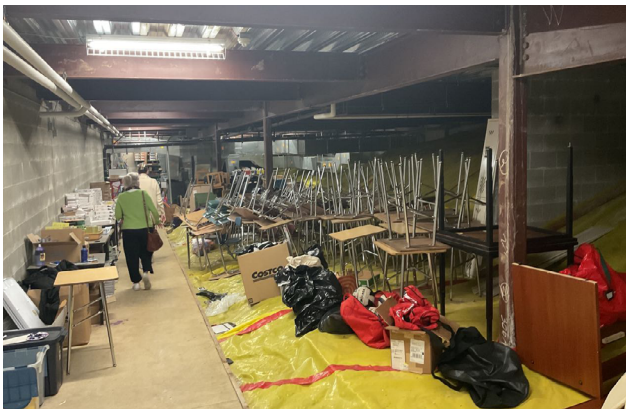
DLR Group image of NKN Middle School's unsprinklered mechanical room - which cannot exist as storage by code.
