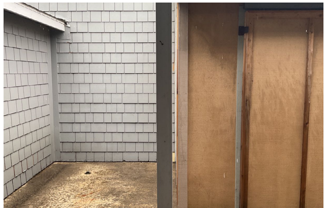
DLR Group image of NKN High School external storage shed, located near the art room.
