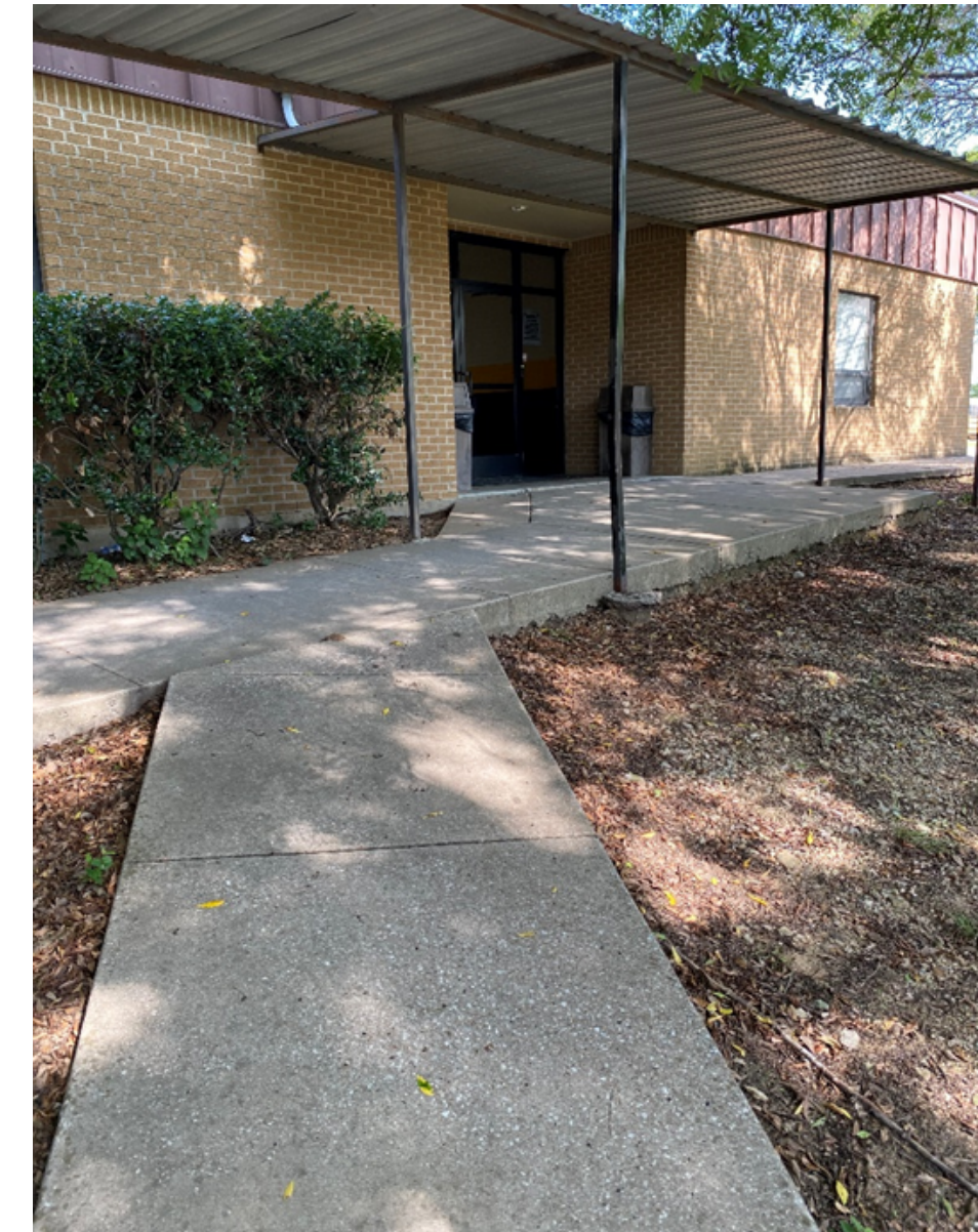
ENTRANCE DOES NOT MEET ADA
