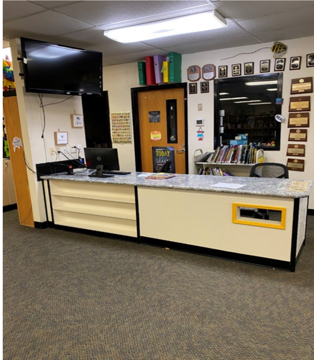
NON-COMPLIANT RECEPTION DESK
