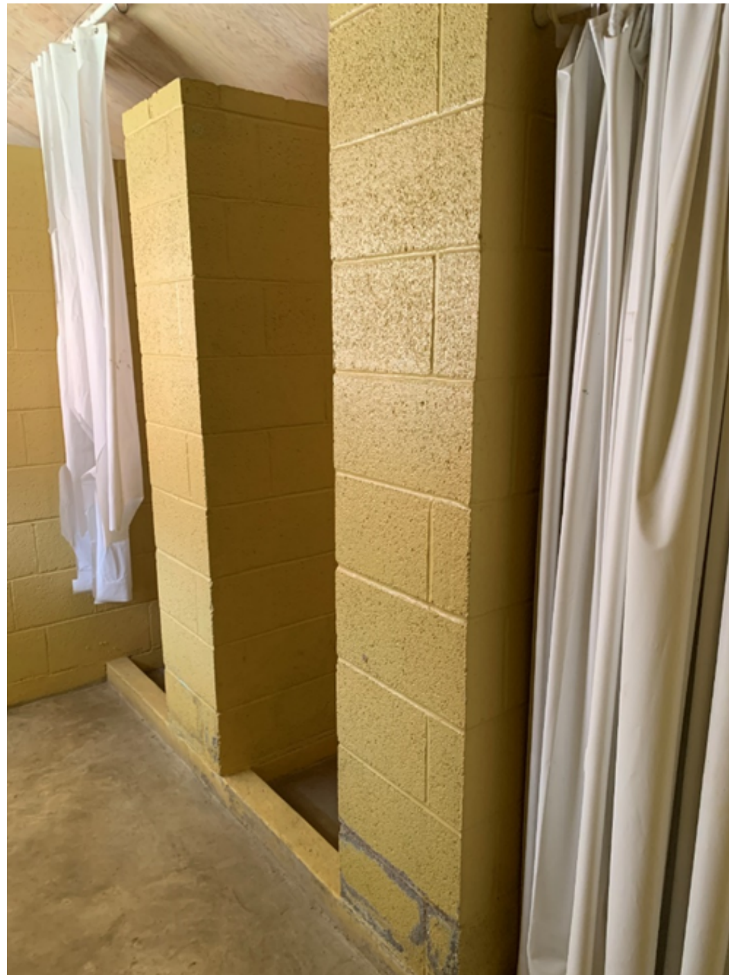
SHOWERS DO NOT MEET TAS/ADA
