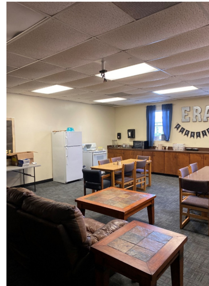
EVIDENCE OF MOISTURE DAMAGE
