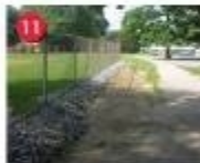
11 Establish Gravel Edge Biofiltration Swale Drainage Area 1 Priority: High Cost: $ Install gravel parking barrier edge to retention structure and outflow. Form and grade structure at biofiltration swale.
