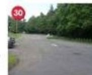
30 Remove Pavement Drainage Area 5 Priority: Low Cost: $0 Convert asphalt road to porous pavement.
