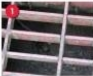
1 Catch Basin Cleaning Energy Disposer Outfall Drainage Area 1 Priority: High Cost: $0 Remove sediment build up within annual catch basins. Provide slope energy dissipator at outfalls.
