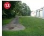
13 Remove Pavement Biofiltration Swale Drainage Area 1 Priority: Med/Low Cost: $0 Remove pavement and convert to biofiltration swale.
