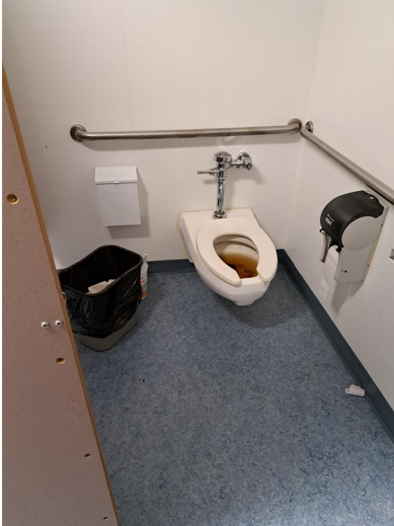
Figure 6 - Restroom of a school that relied on teachers cleaning
