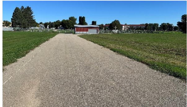
Photo 1: Worn Track Surfacing
