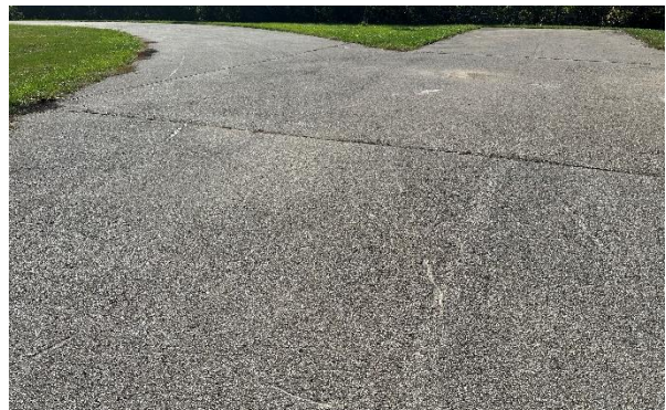
Photo 3: Longitudinal and Transverse Cracking
