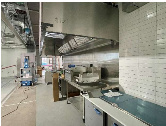
Kitchen Equipment Installed
