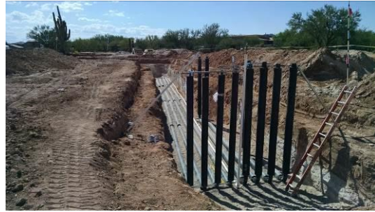
Chiller Pipes From 200 Bldg to 300 Bldg
