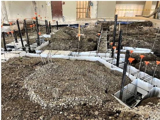
Void Boxed Plumbing in Kitchen Area
