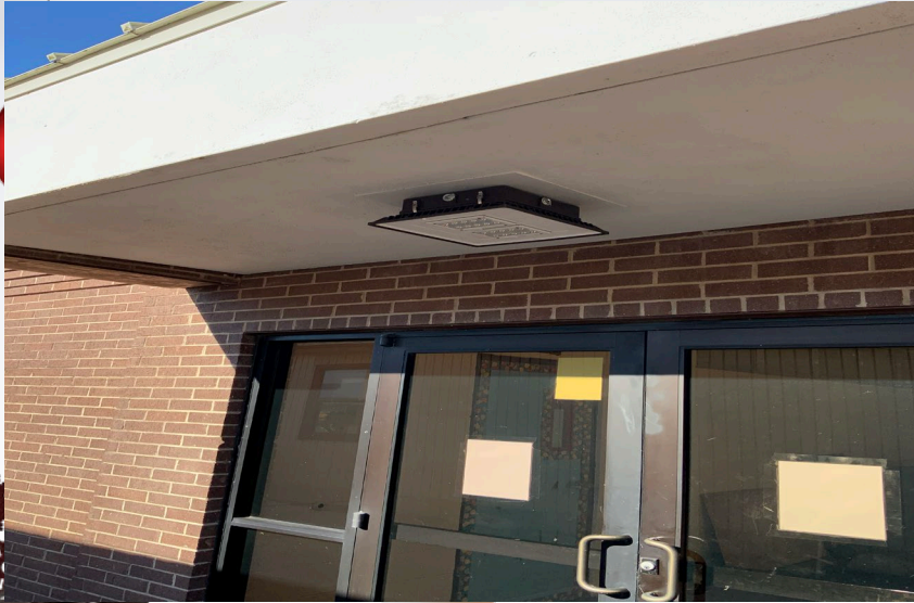
Wall Packs, Exterior light
