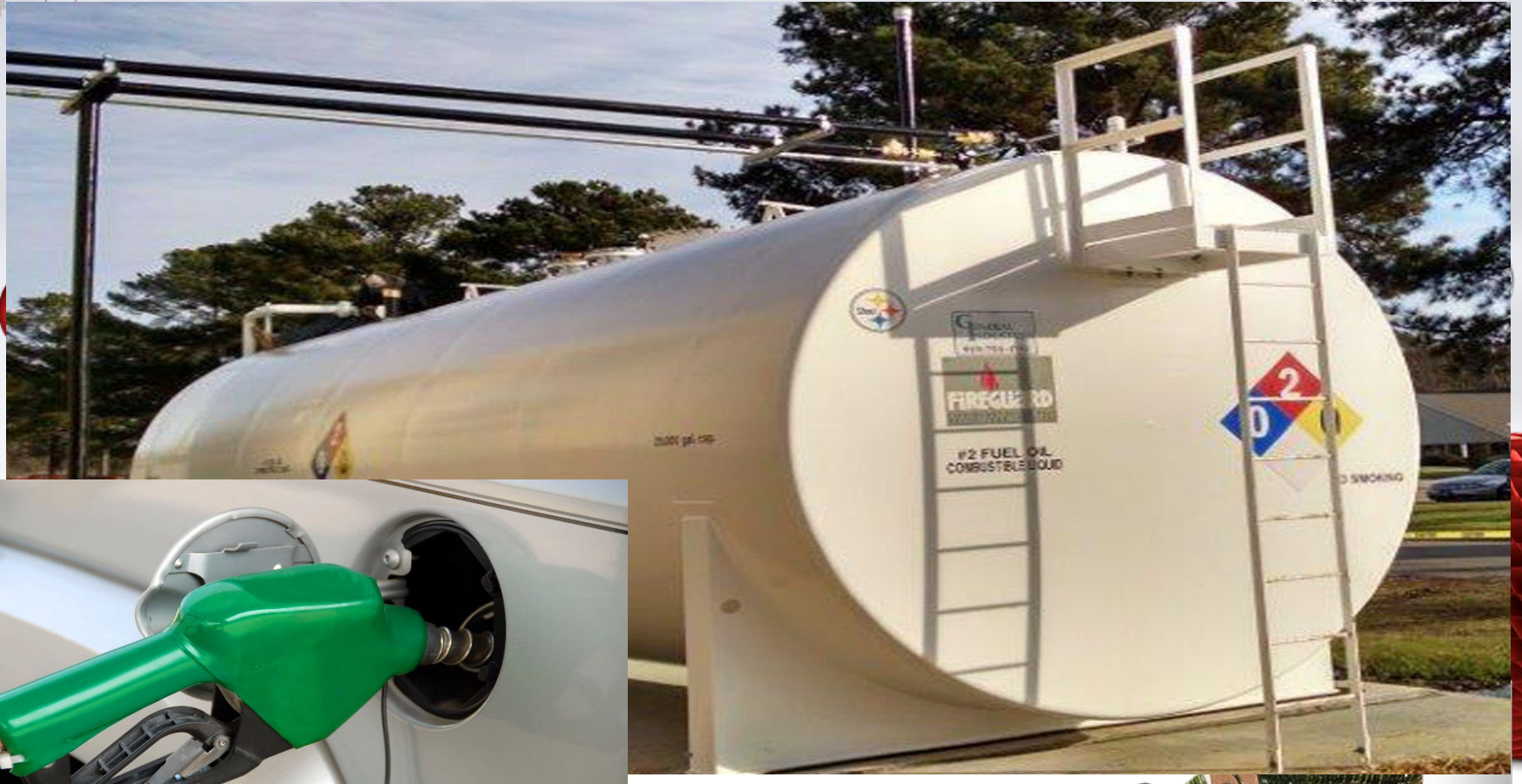
Above Ground Fueling Station
