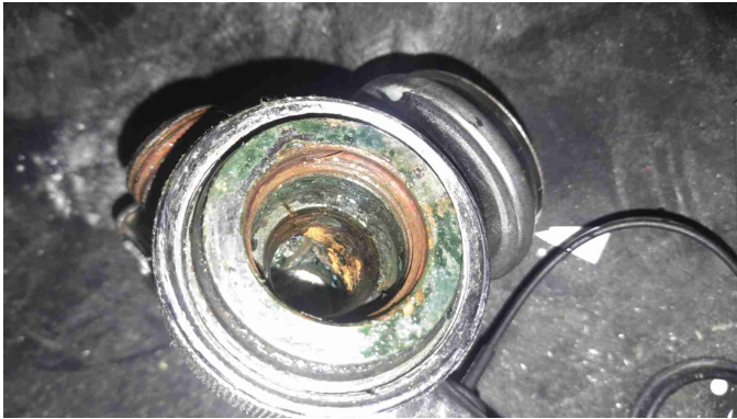
FE #3 - Bad Valve Assembly
