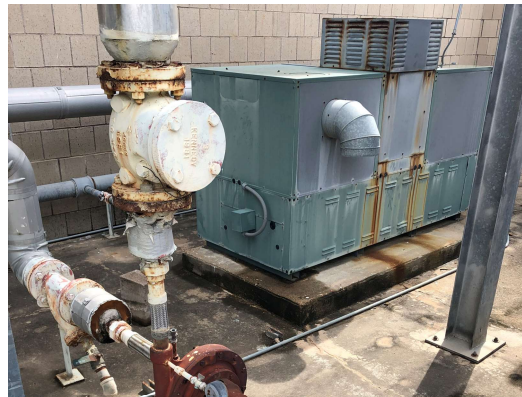
Junior High Boiler
