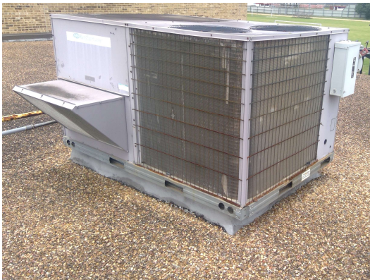
High School RTU
