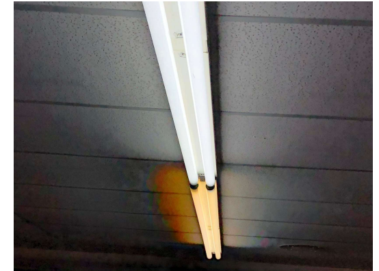
Retrofit Fluorescent Lamps
