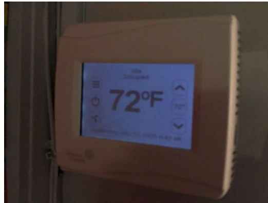
RCx Existing JCI Controls
