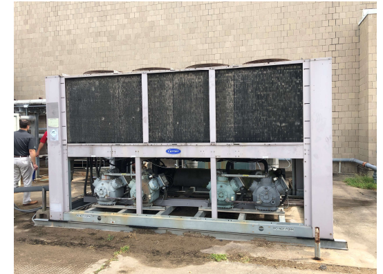
Junior High Chiller
