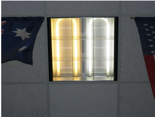
Retrofit Fluorescent Lamps
